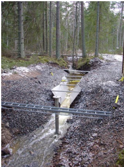
Figure A1-2. Top: Before cleaning of vegetation in Sep. 2004. Middle: After excavation and refilling with crushed stone and gravel, Sep. 2004. Bottom: After installation in Jan. 2005, the screened tube with devices for measurement of electrical conductivity and temperature in the foreground.
