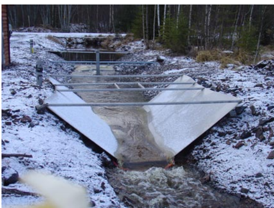
Figure A1-1. Top: Winter conditions in Feb. 2004 before reinstallation. Middle: Reinstallation in Oct. 2004. Bottom: After reinstallation, winter discharge in Jan. 2005 exceeding the capacity of the small flume.
