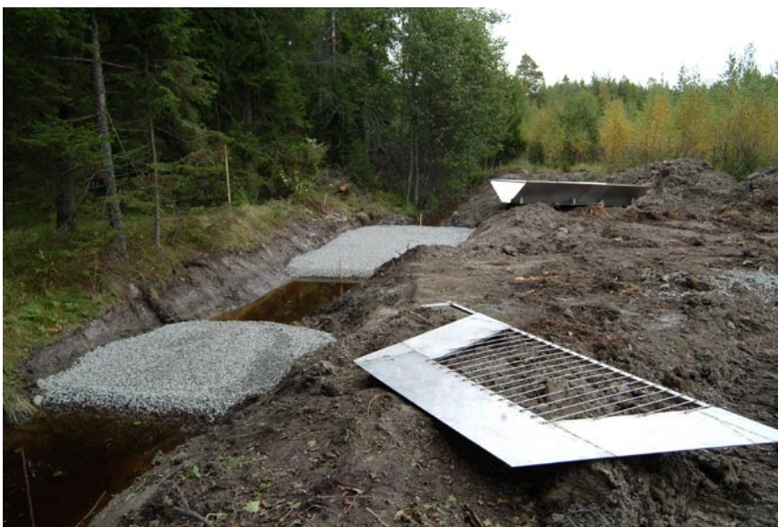
Figure 4-2. Excavation of the reach of the brook and the foundation for the flumes (excluding the top sand layer) at PFM002667. In the foreground the iron bars installed upstream the flumes to avoid disturbances of debris can be seen.
