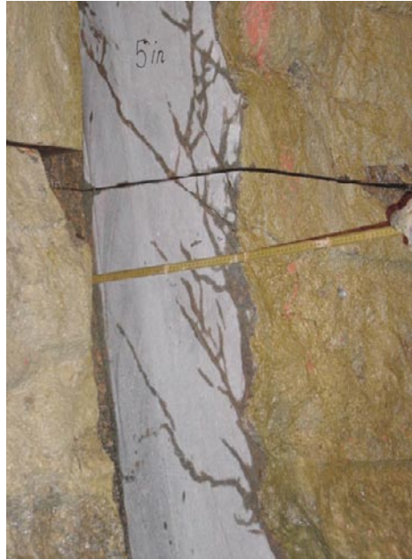
Figure 7-17. Open cracks in the right slot wall.
