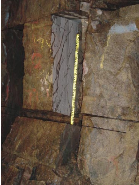
Figure 7-10. Cracks from left slot wall.
