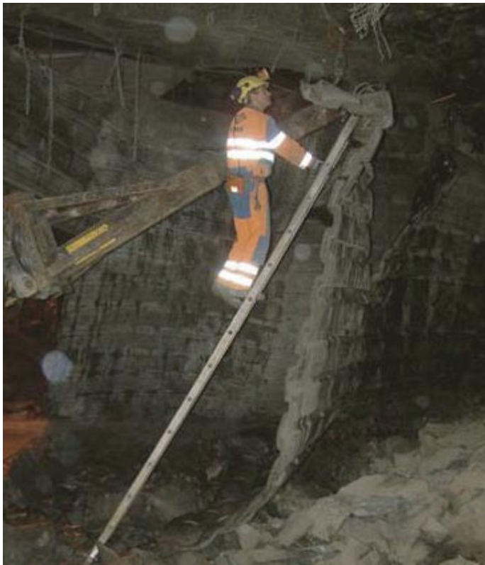
Figure 3-2. The restrictions on damage in the main tunnel, as well as the limited working hours caused the need for extensive safety measures during excavation of the first roughly 16 m of the tunnel. The photo shows installing a rubber mat for fly rock protection. Notice shape and size of the mucked rock in the lower right part of the photo.
