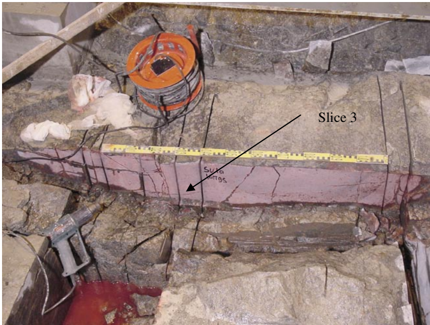
Figure 7-34. A saw cut along the tunnel direction.
