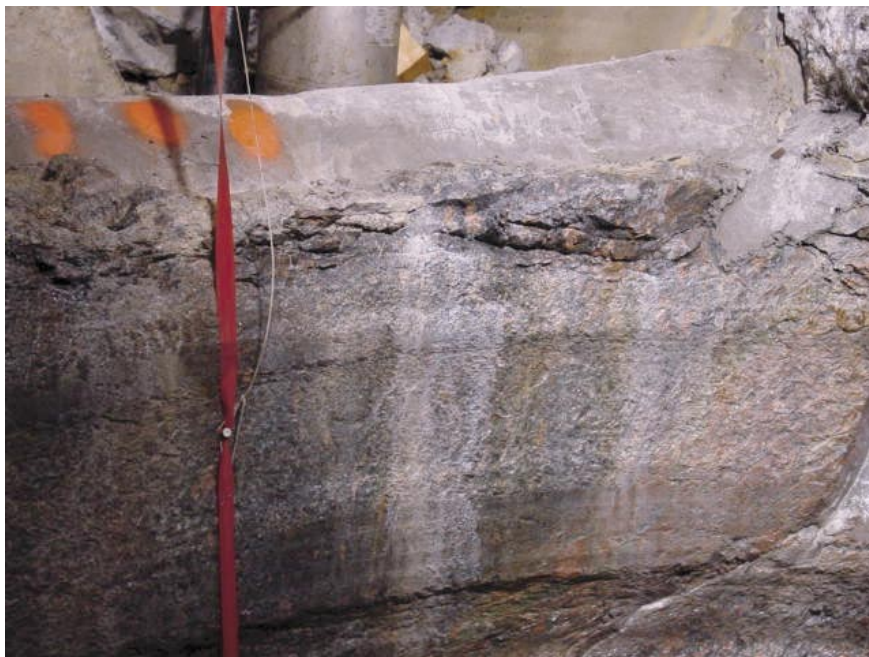
Figure 7-4. Observations of the upper part of a 1.8 m diameter bore hole. The upper part is a concrete slab that was casted to provide a smooth surface for collaring of the bore hole. The slab is approximately 0.3 m thick.
