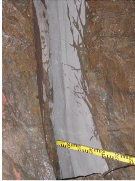
Figure 7-21. Cracks from the tunnel and bench.
