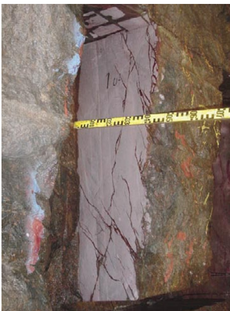
Figure 7-12. Cracks from right slot wall.
