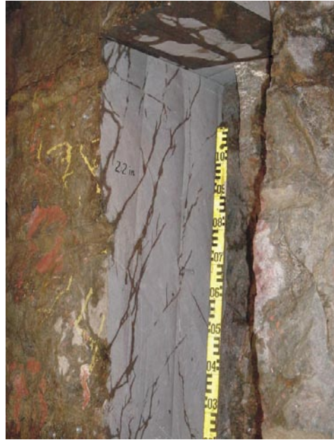
Figure 7-11. Cracks from upper part of left slot wall.
