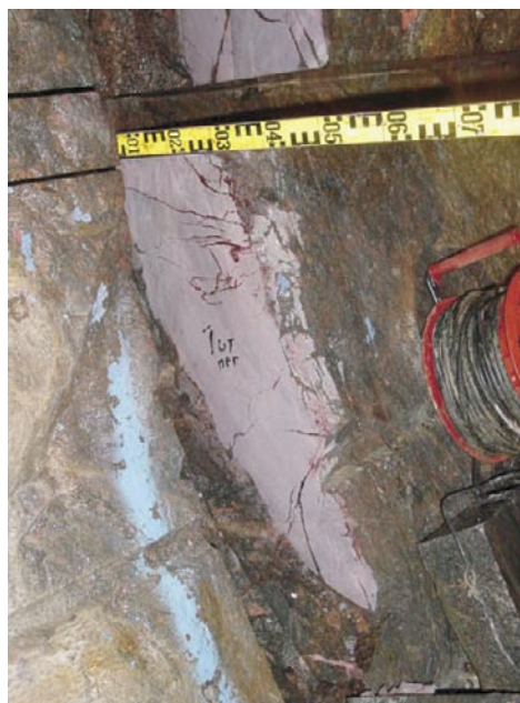
Figure 7-13. Cracks from the bench, right slot wall.
