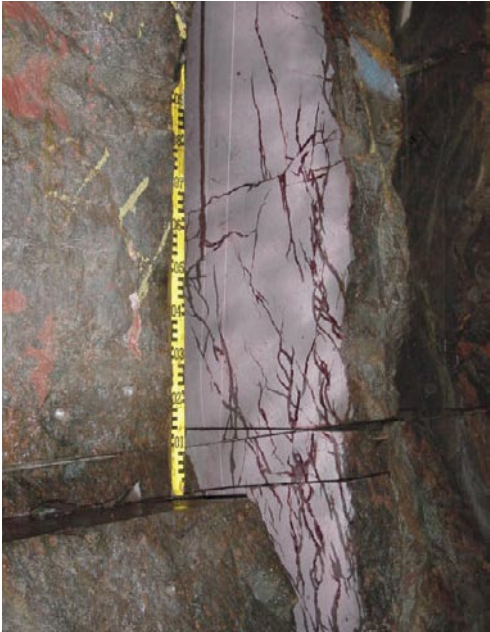
Figure 7-9. Cracks in lower part of right slot wall.
