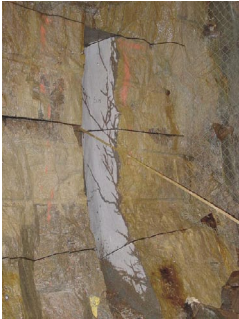
Figure 7-16. Cracks from the right slot wall.
