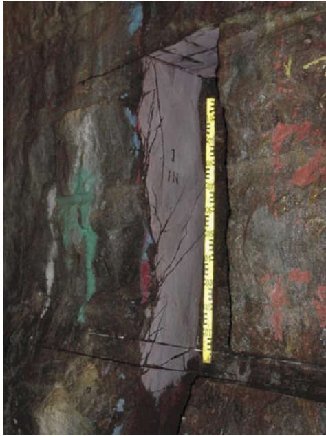
Figure 7-14. Cracks from left slot wall.
