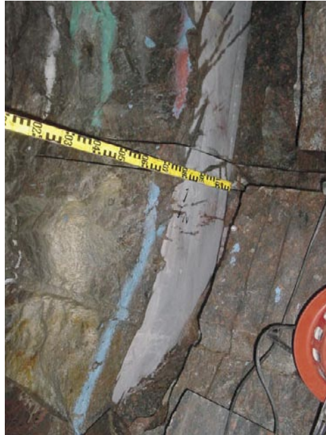
Figure 7-15. Cracks from the bench, left slot wall.
