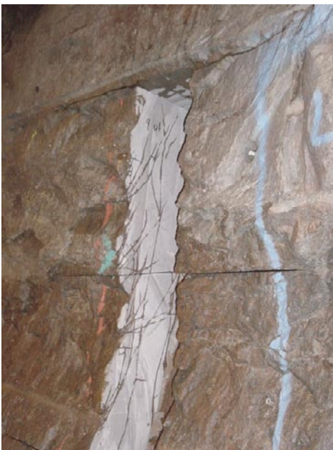
Figure 7-22. Cracks in the left wall.
