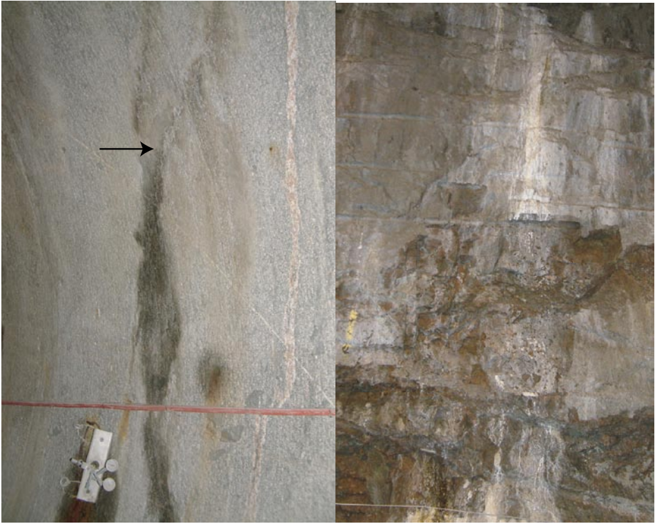
Figure 2-3. The waterbearing fracture set 2, trending NW. Observation in the TBM tunnel just outside the TASQ tunnel (left). Notice how the fracture spays into two in the upper part of the photo. The right photo is from the TASQ tunnel. The fracture set is perpendicular to the tunnel, and (at the arrow) less visible. This section was grouted, the light strips are calcite precipitation from the cement.
