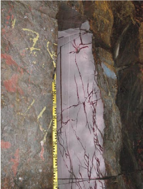
Figure 7-8. Cracks in upper part of right slot wall.
