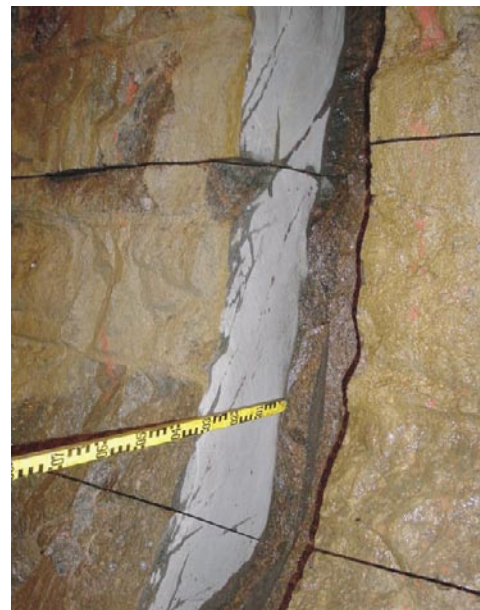
Figure 7-19. Cracks from the left slot wall.
