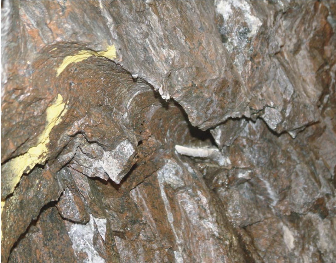
Figure 6-8. A grout hole at section 0/050.7, location is indicated in Figure 6-7. The white slab in the bottom of the borehole is cement from the grouting. The hole was not fully filled with the grout slurry, and the cement has sedimented in the hole. Borehole diameter is 64 mm.
