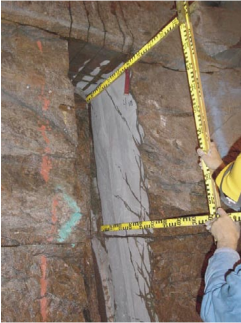
Figure 7-20. Cracks from right wall.
