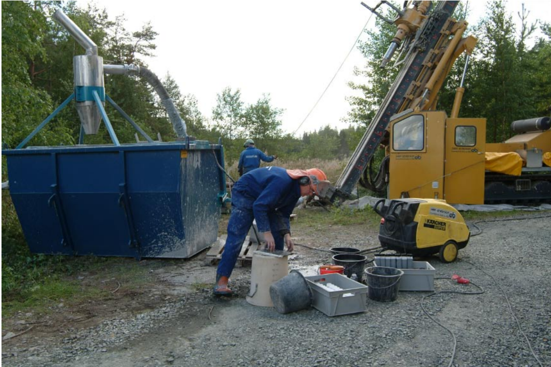
Figure 3-5. To improve flow measurements and simplify sampling of soil, drill cuttings and groundwater, a new container with a specially designed cyclone was used during drilling of HFM20–22.
