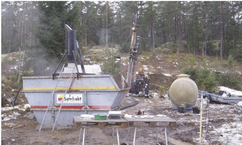
Figure 4-2. Return water from drilling (HLX30) is led to a settling container. The cyclone for collecting the cuttings can be seen fastened on top of the container. Equipment for the preliminary geological logging can be seen in the foreground.
