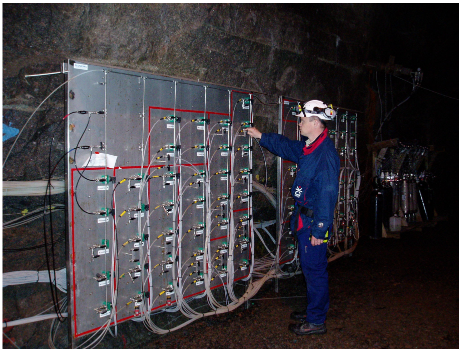
Figure 6-4 Panel with pressure transducers in tunnel G
