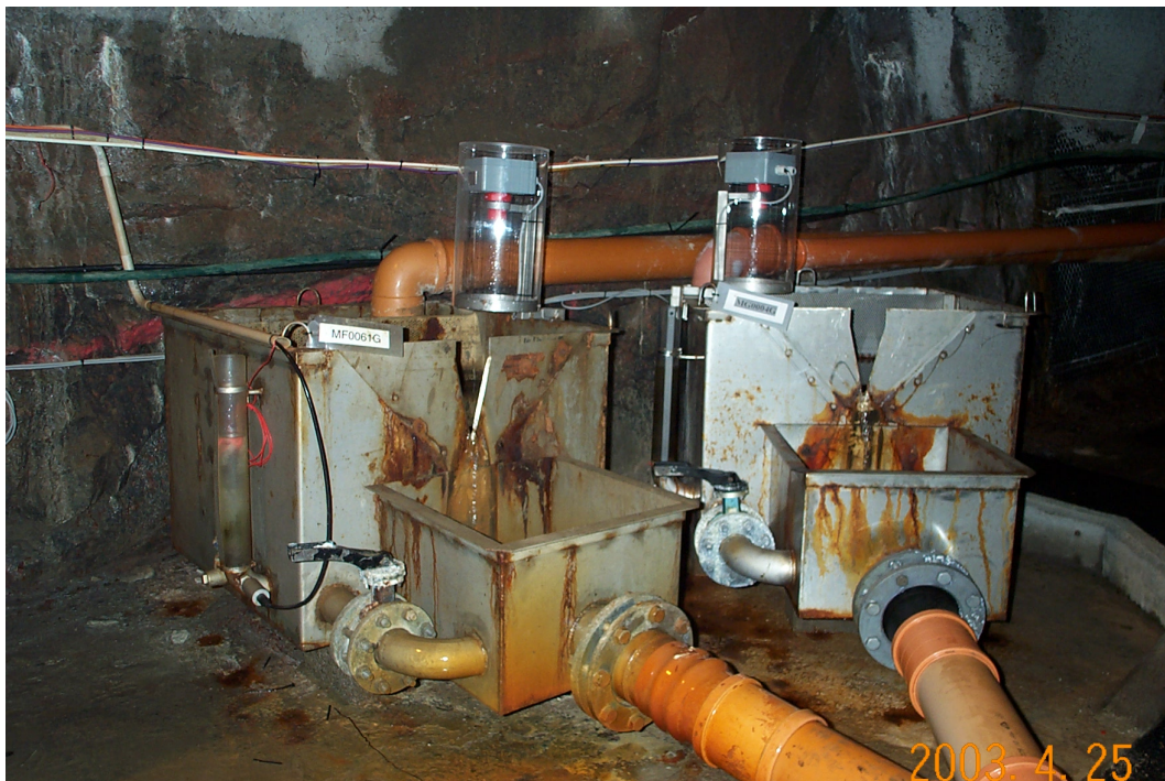
Figure 5-6 Measurement units for MF0061G and MG0004G at PG5
