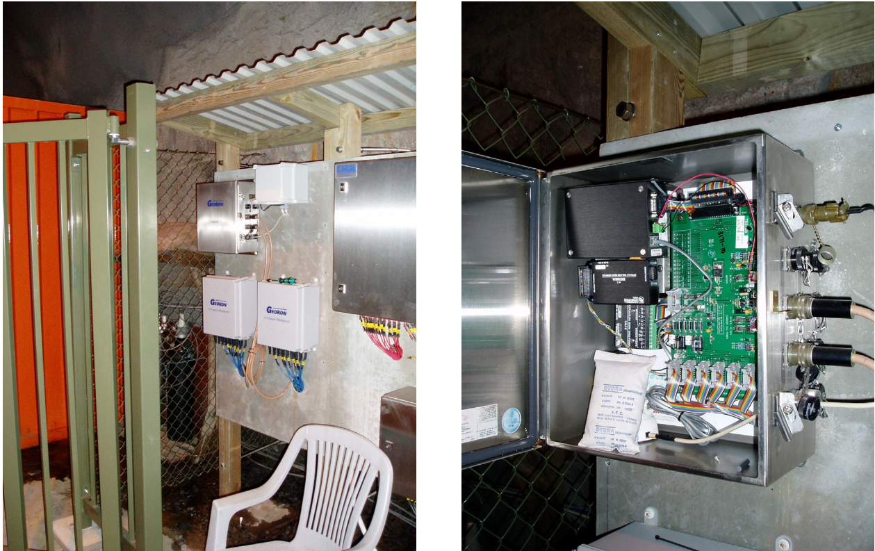
Figure 4-3 Data loggers for the Hydro Mechanical equipment, located in Tunnel G.
