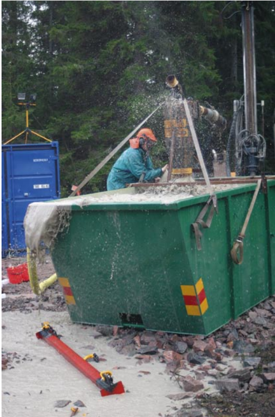
Figure 3-32. Percussion drilling of HFM16, whereby an inflow of groundwater to the borehole of 1,200 l/min was measured.
