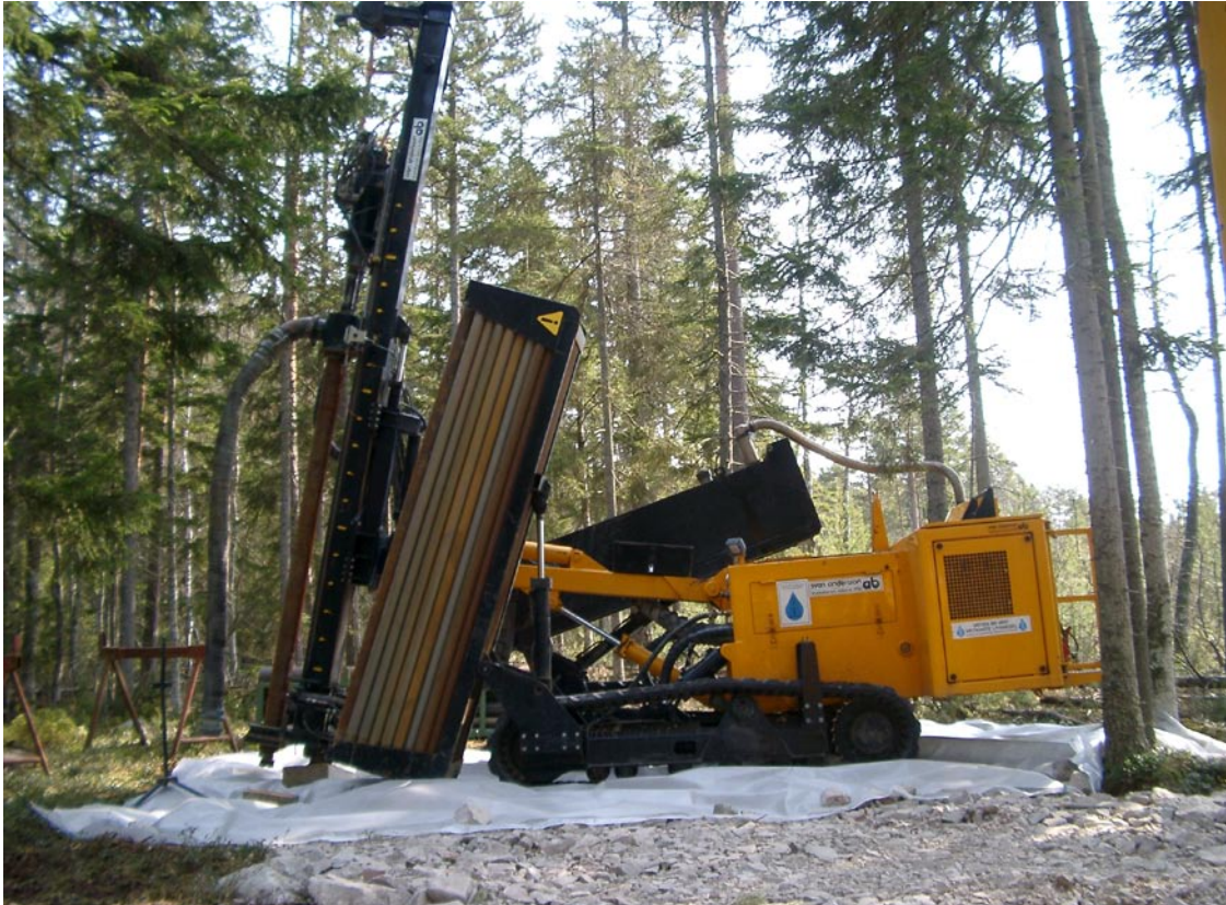
Figure A-5. Percussion drilling machine set up on protective ground cloth that prevents ground contamination and permits any leakage to be collected.
