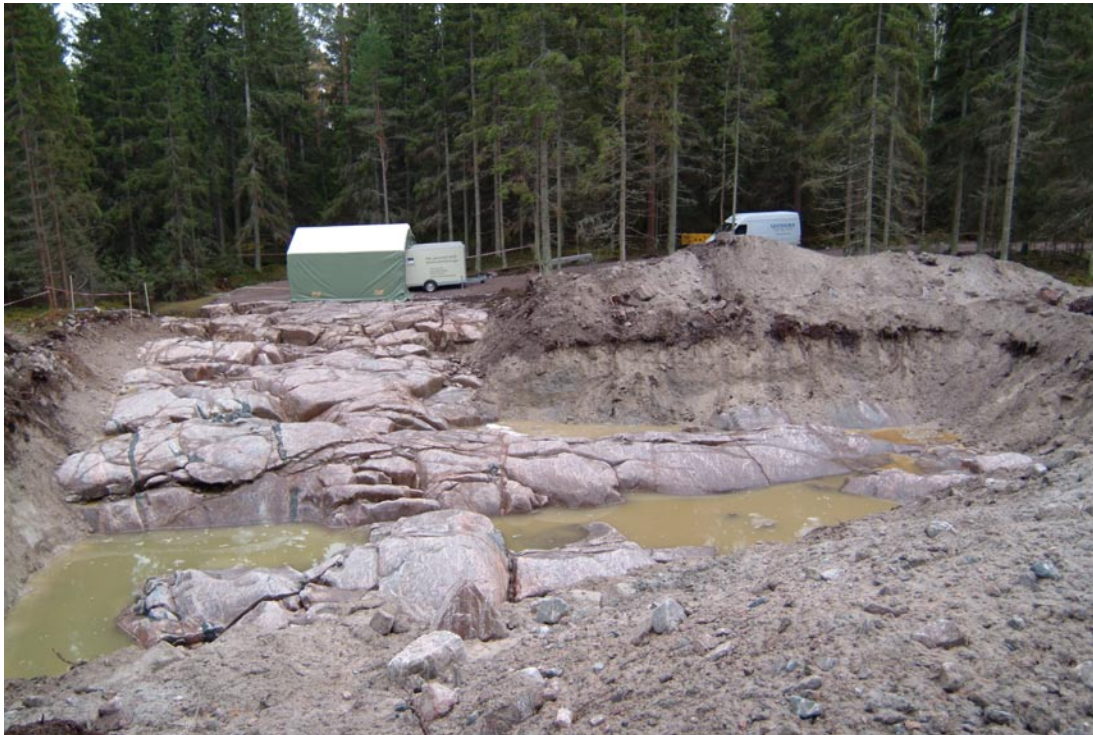
Figure 1-3. The excavated area at drilling site DS5 with the highly fractured bedrock surface.
