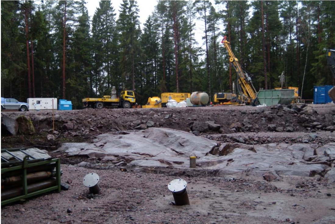
Figure 1-4. Percussion drilling of KFM05A on DS5, with percussion boreholes HFM14 (right) and HFM15(left) as well as HFM14B (yellow cap) in the foreground.
