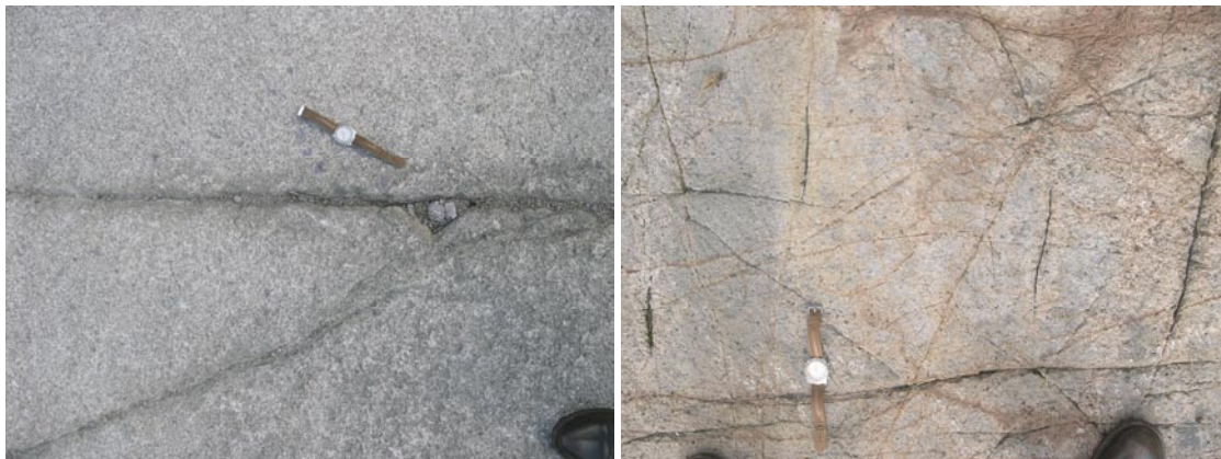
Figure 5-4. Qualitative difference in fracture networks between the outcrop ASM000025 (left), and ASM000205 (right). The density of small fractures is much larger in the latter than in the former.
