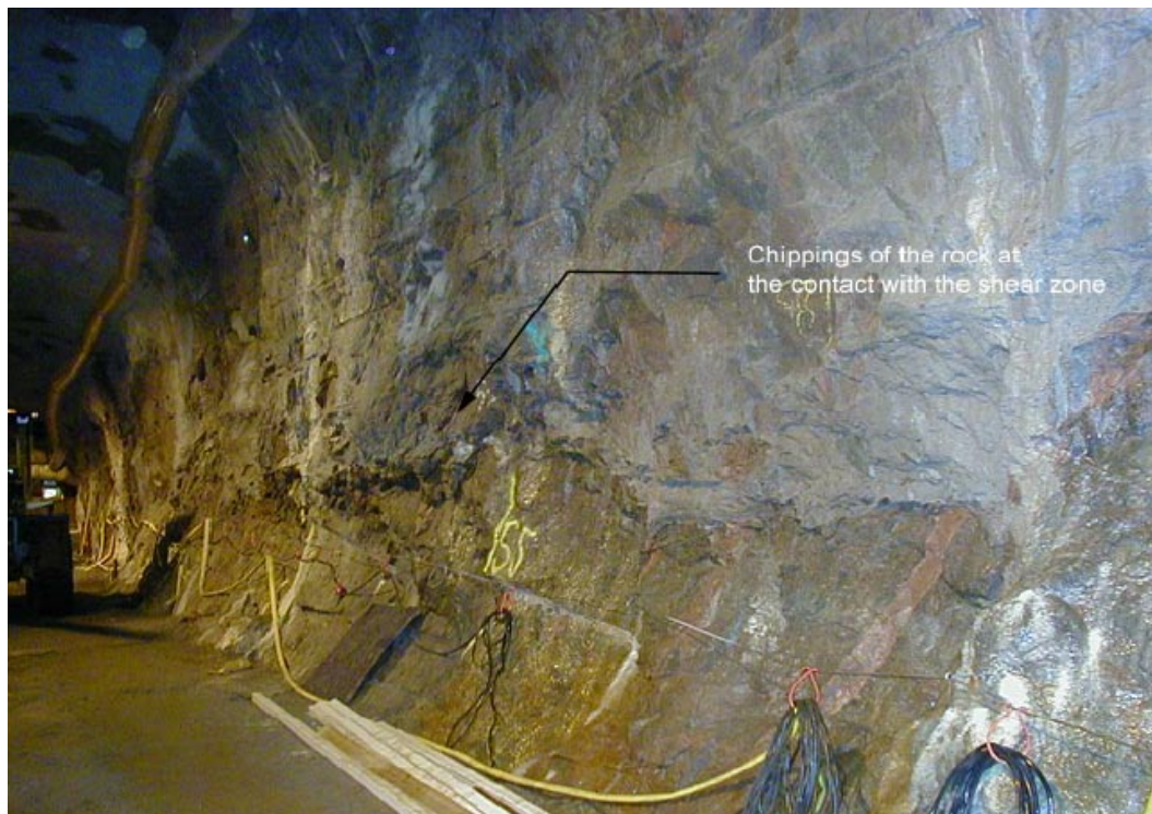
Figure 3-5. Overview of the “chippings” on the west wall of the tunnel. The chipping is intensified due to blasting damage in the floor of the pilot drift which was located at the approximate same depth.
