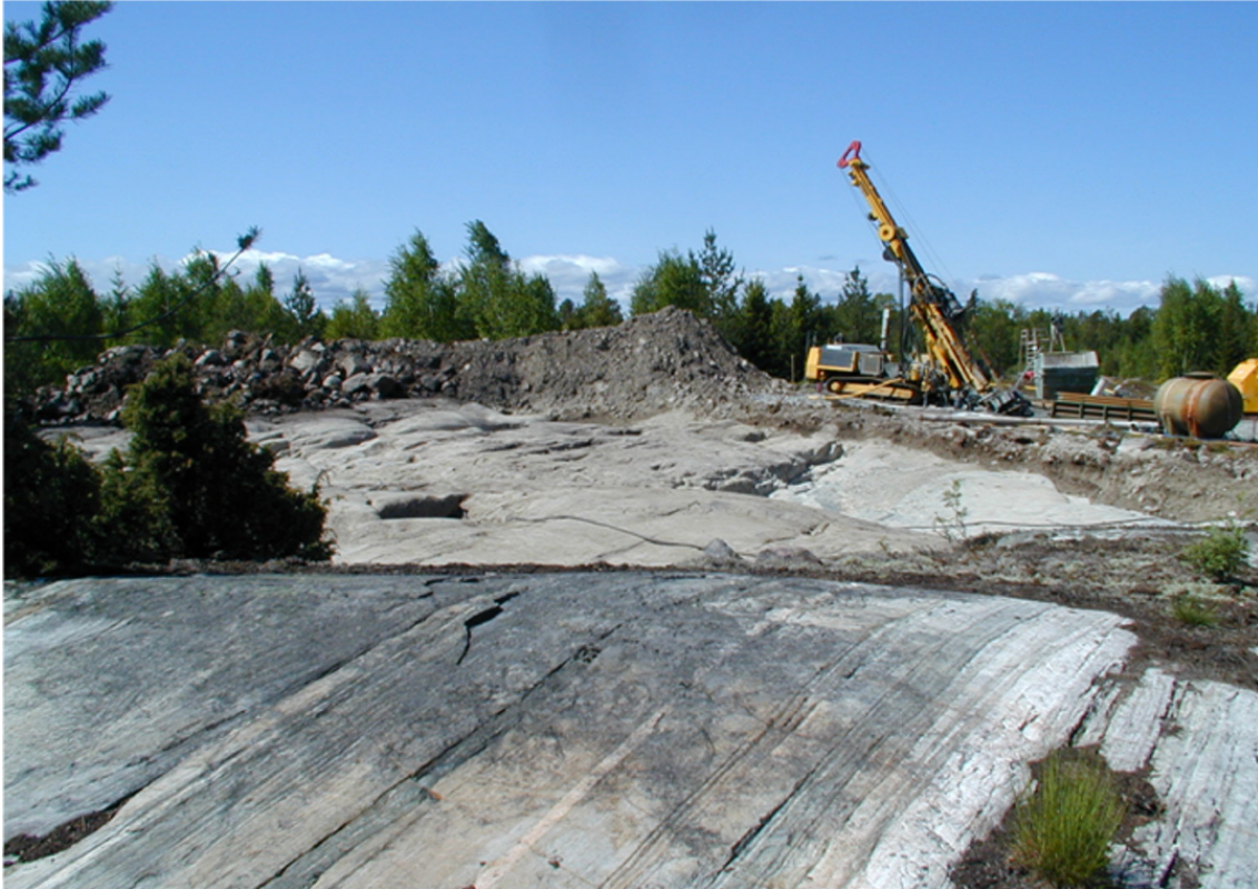
Figure 5-1. Photo from trenching at Drill Site 4 at Forsmark for the purpose of mapping
