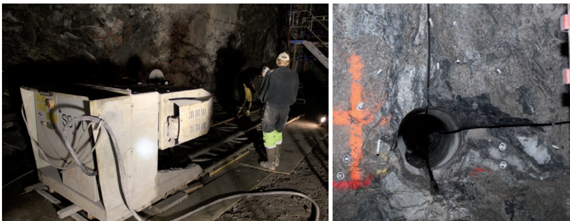
Figure 3-5. Photo of the equipment for driving the diamond wire and to the right there is a close-up picture of the lower corner hole after the sawing has been made.
