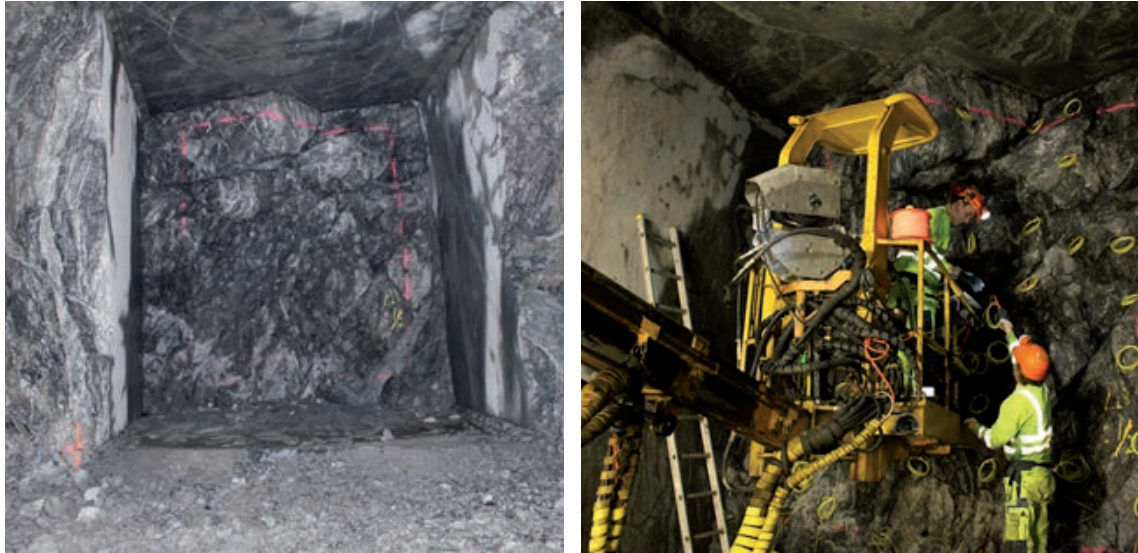
Figure A1-4. Photo of the front facing round No 2 and to the right is the charge of round No 2
