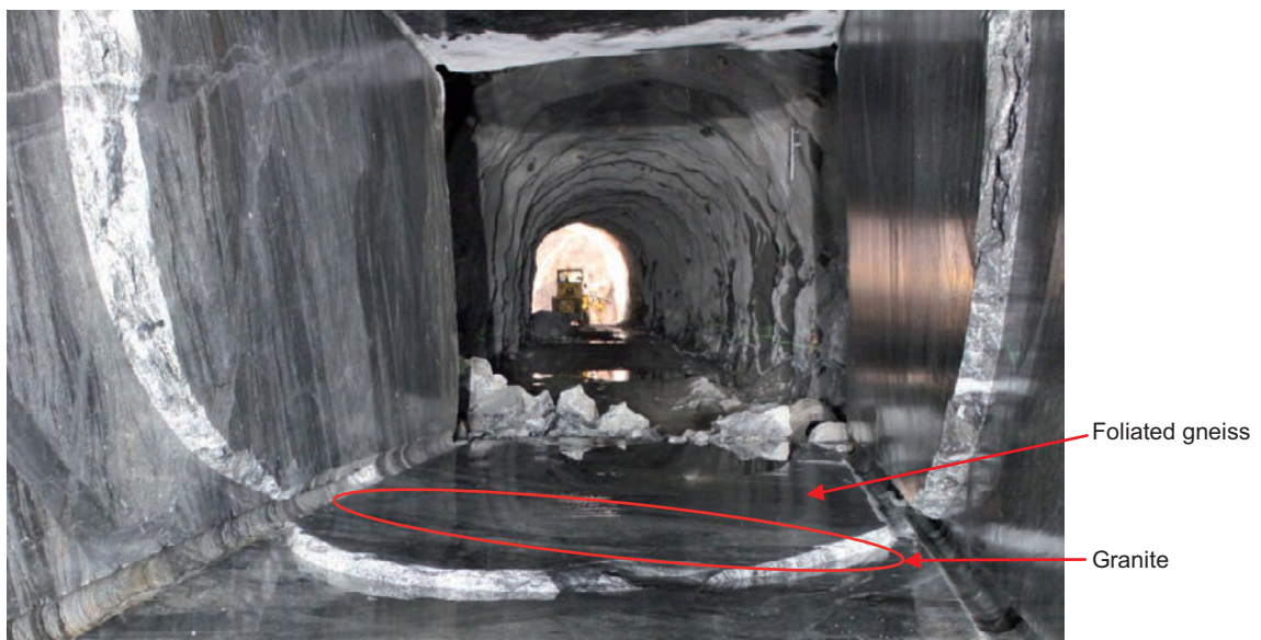
Figure 5-10. Detail of the tunnel floor in phase 2 where ground radar measurements were made. The rock varies from granite to foliated gneiss.
