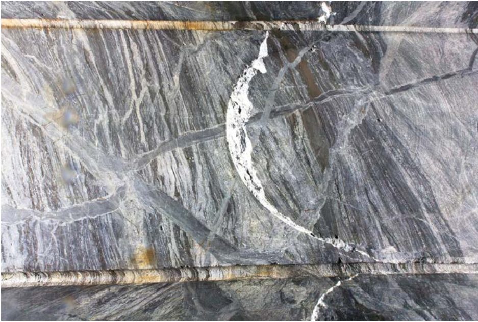
Figure 5-3. Detail of the finished blasted tunnel, the left wall at the transition between the two phases.
