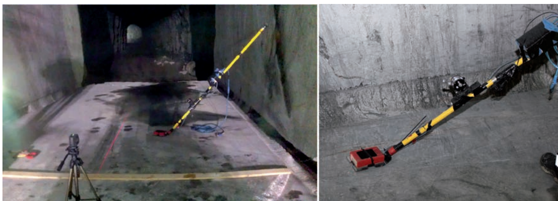
Figure 5-8. Image of the measurement area of ground penetrating radar (left) and an image of the measuring device (right).
