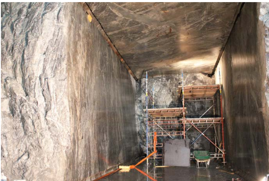
Figure 4-2. Phase 2 – In order to perform the drilling of the holes on the upper level, the construction of fixed scaffolds and platforms was required. In the actual production of deposition tunnels, the fixed platforms will be replaced with mobile lifting platforms to achieve a rational work.
