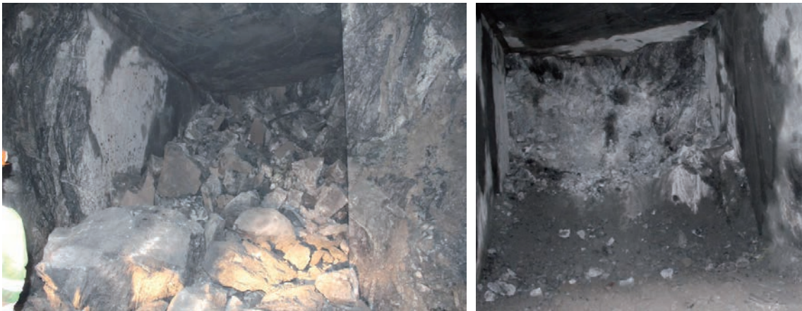
Figure 4-5. The left photo shows the face after blasting of round No 2 and the photo on the right shows the face after removal of the loos rock material.
