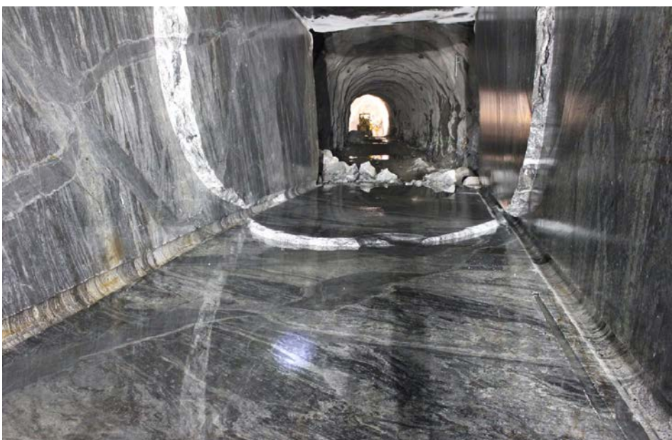
Figure 5-2. Detail of the finished blasted tunnel. The light field is the step between phase 1 and 2.
