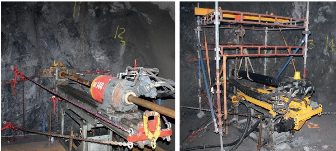
Figure 4-1. Phase 1 – The left image shows the drilling of the core drill hole \text{Ø } 76 \text{ mm} . By changing the boom on the drilling unit (right picture) the reaming of the borehole core in two steps was made, from \text{Ø } 76 \text{ mm} to \text{Ø } 165 \text{ mm} , then from \text{Ø } 165 \text{ mm} to \text{Ø } 255 \text{ mm} . No new scaffold was required for these reaming steps.
