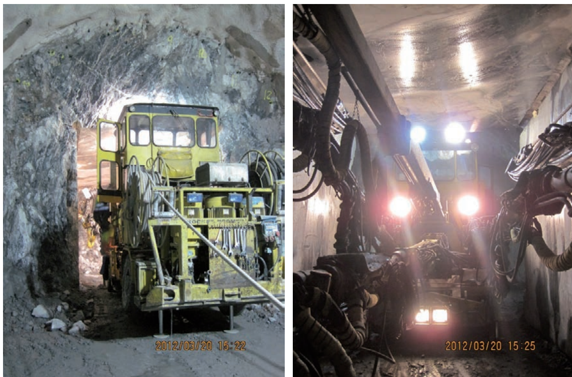
Figure A1-1. The drilling unit for the drilling of holes for blasting – Atlas Copco Rocket Boomer 353.
