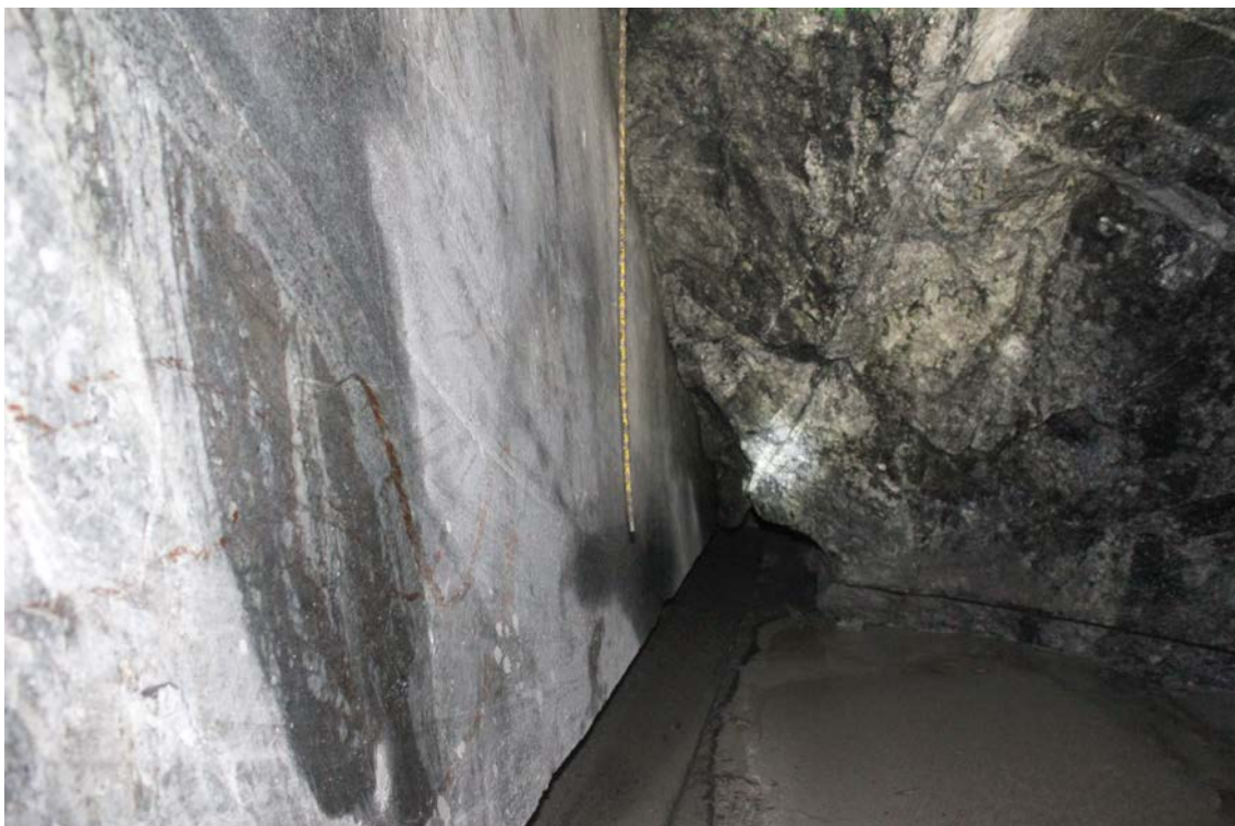
Figure 4-3. During the sawing in phase 2 a break of diamond wire occurred (vertical yellow line in the middle of picture at the rock surface).
