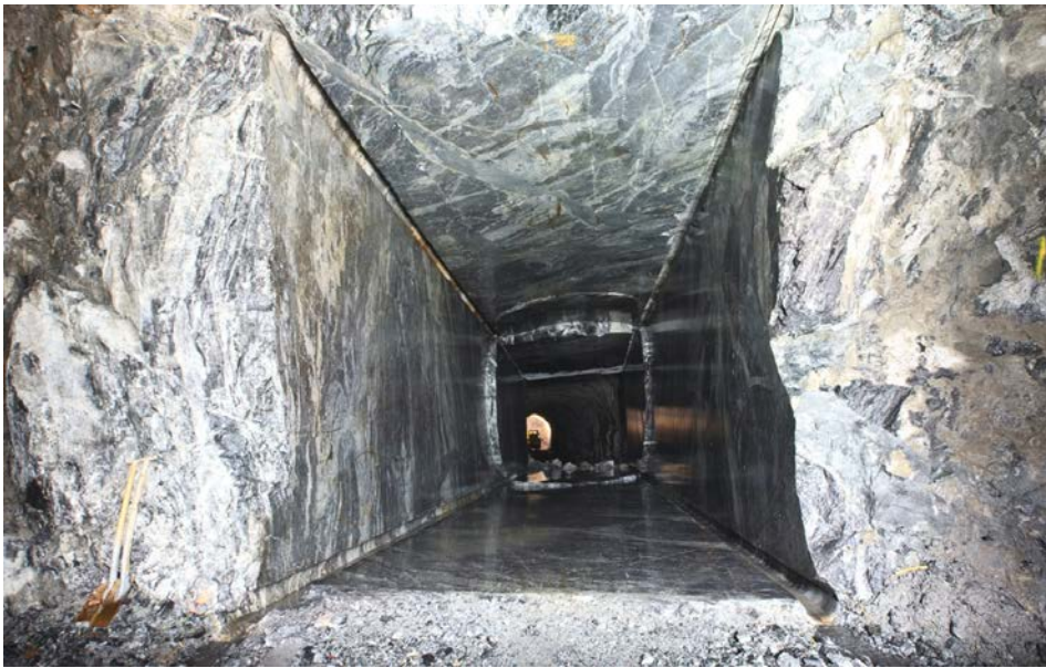
Figure 5-1. Overview photo of the finished blasted tunnel, phase 1 closest to the camera.
