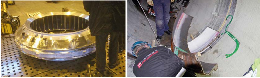
Figure 4-23. To the left a picture from the compartment plug FAT and to the right the installation of the plugs fastening ring.
