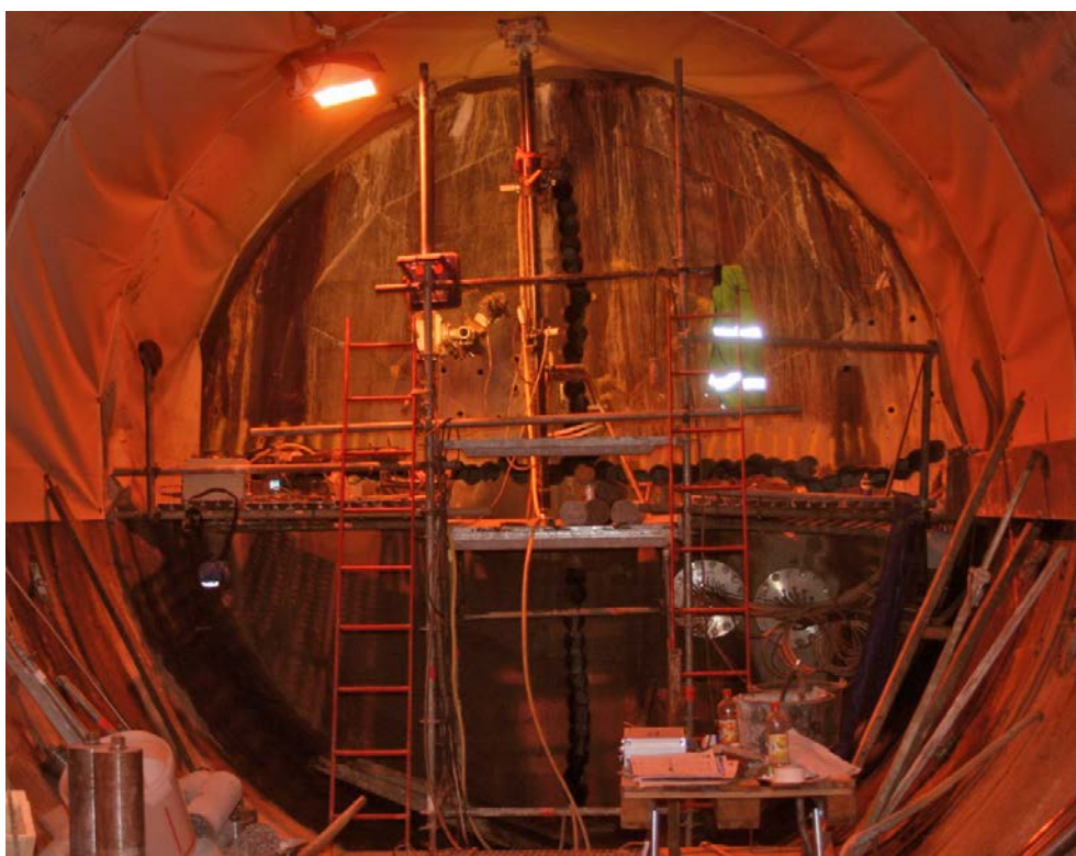
Figure 4-4. Breaching of the outer plug in December 2010 with the core drilled holes before hydraulic splitting.
