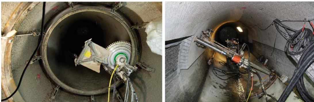
Figure 4-22. The picture to the left illustrates the sawing of a compartment plug notch and to the right a picture from drilling of sensor holes. The right picture also illustrates the sawed out cable notches on both sides of the drift, these will be partially casted after the piping is installed.
