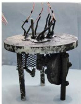
Figure 4-33. As the result of microbial activity and corrosion of cast iron, a precipitate of iron sulphide has formed on the instruments mounted inside the support cage.
