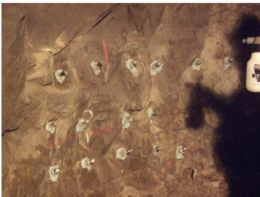
Figure 7-18. Mounted rock bolts in the Äspö tunnel are salt sprayed once a month during a period of one year.
