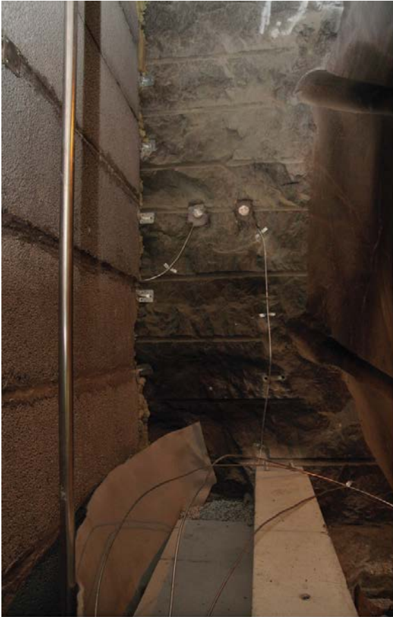
Figure 4-44. Detail photo showing (from left) filter of leca-beams and macadam, drainage (air) pipe, geotextile, bentonite seal of MX-80 (blocks and pellets) and concrete delimiters. All sensor cables are led in steel tubes.
