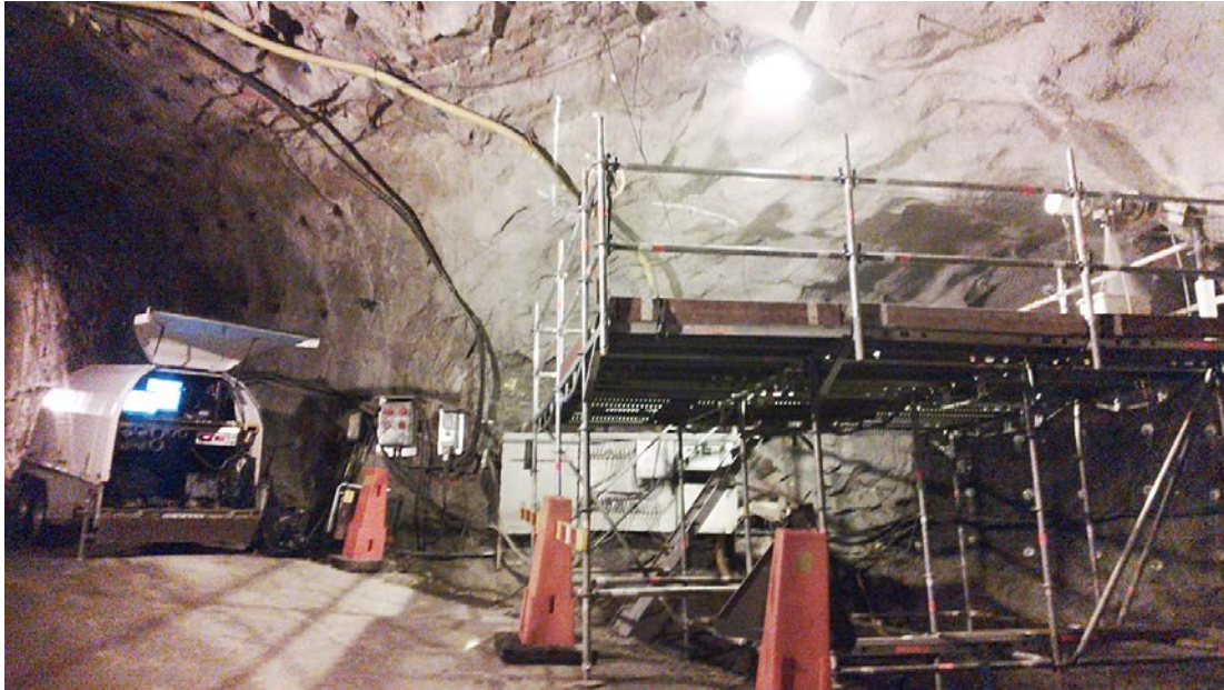
Figure 5-1. Measurement trailer mobilised at KA3011A01.
