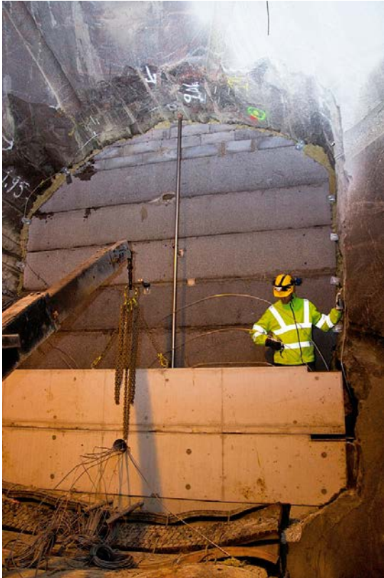
Figure 13-10. Installation of concrete beams that comprise the inner form wall for the concrete dome in a full-scale test of the complete plug system. A bentonite seal, crushed rock, filter and sensors are installed behind the concrete beams.
