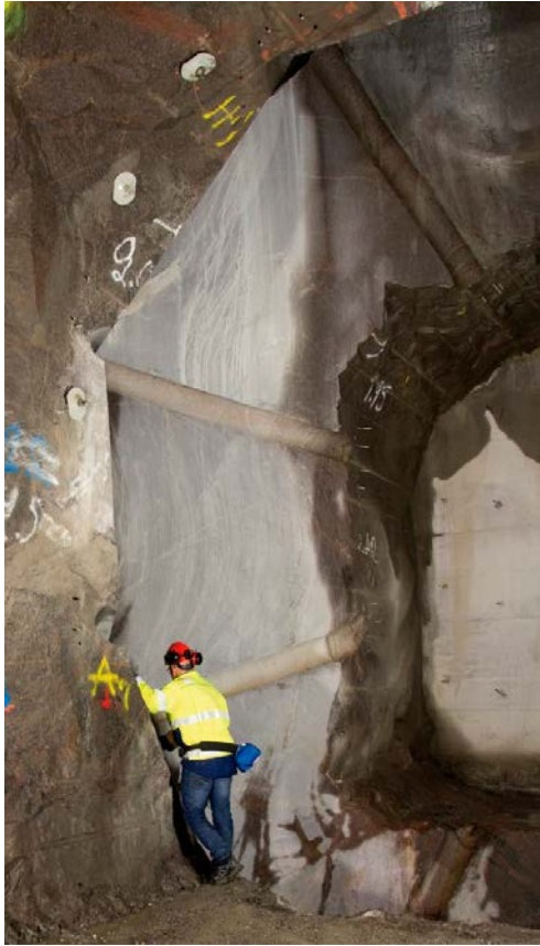
Figure 13-11. Inspection of wire-sawn slot for the concrete dome in the full-scale experiment. Left side of experimental tunnel TAS01 (see Figure 13-8).
