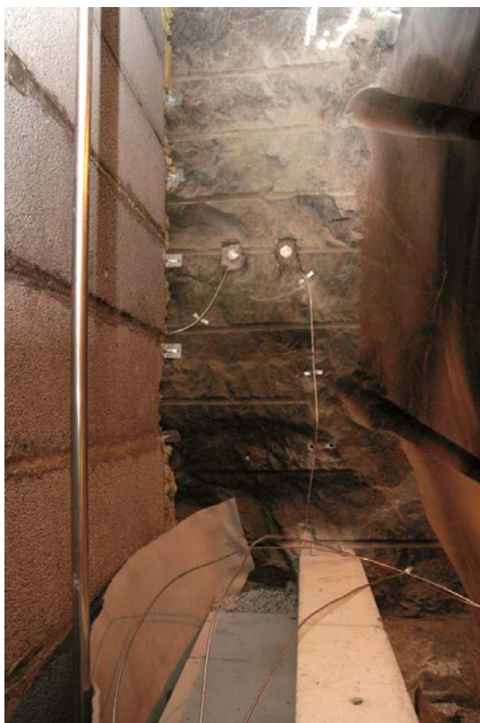
Figure 13-9. Detail photo from the installation of the full-scale test of the complete plug system. The picture shows (from left): filter of Leca beams and crushed rock, drainage pipe (air evacuation), geotextile, bentonite seal with MX-80 clay (blocks and pellets) and concrete beams. All sensor cables are run in steel tubes on the pressure side of the experiment.
