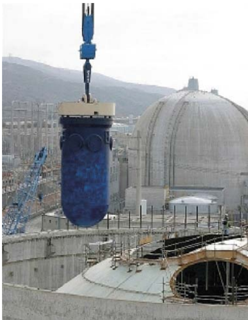
Figure A1-28. Removal of the San Onofre RPV via the reactor containment.
