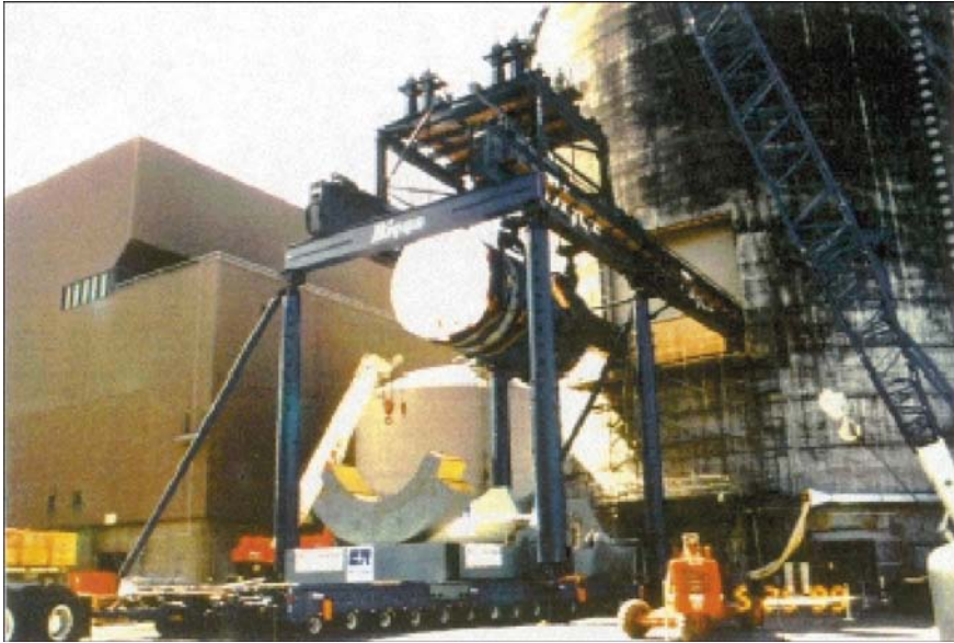
Figure A1-29. Removal of the Big Rock Point Pressure Vessel via a new side access.
