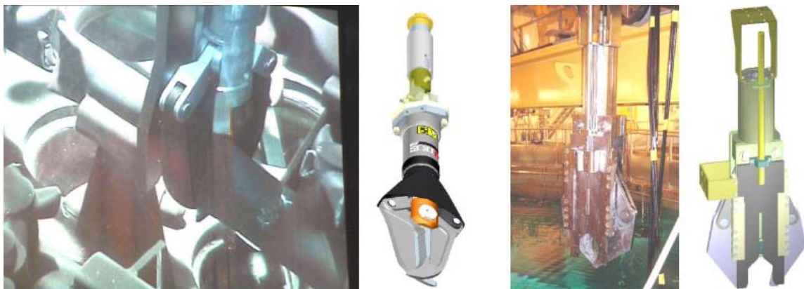
Figure A1-1. Shearing tools used to cut the core spray system and flat bars on the core grid.
