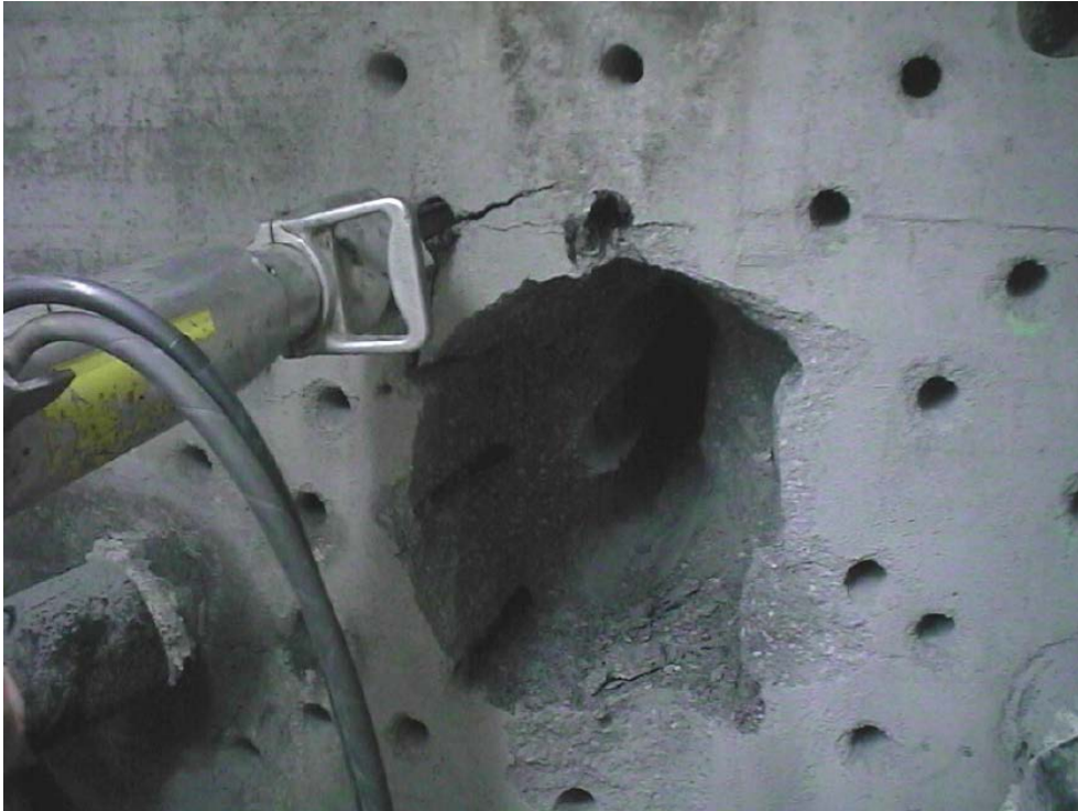
Figure A-38. Breaking pattern concentric to free surface. Hydraulic splitter in operation (Bárcena et al. 2003).
