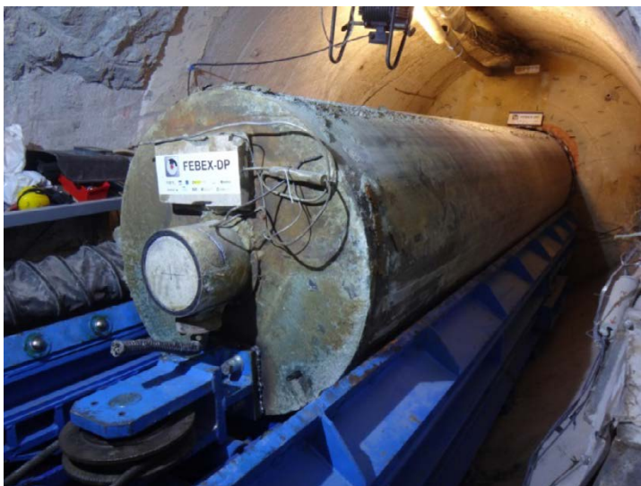
Figure B-7. Extraction of heater #2. View of the extracted heater, part of the extraction vehicle and the return pulley (García-Siñeriz et al. 2016).
