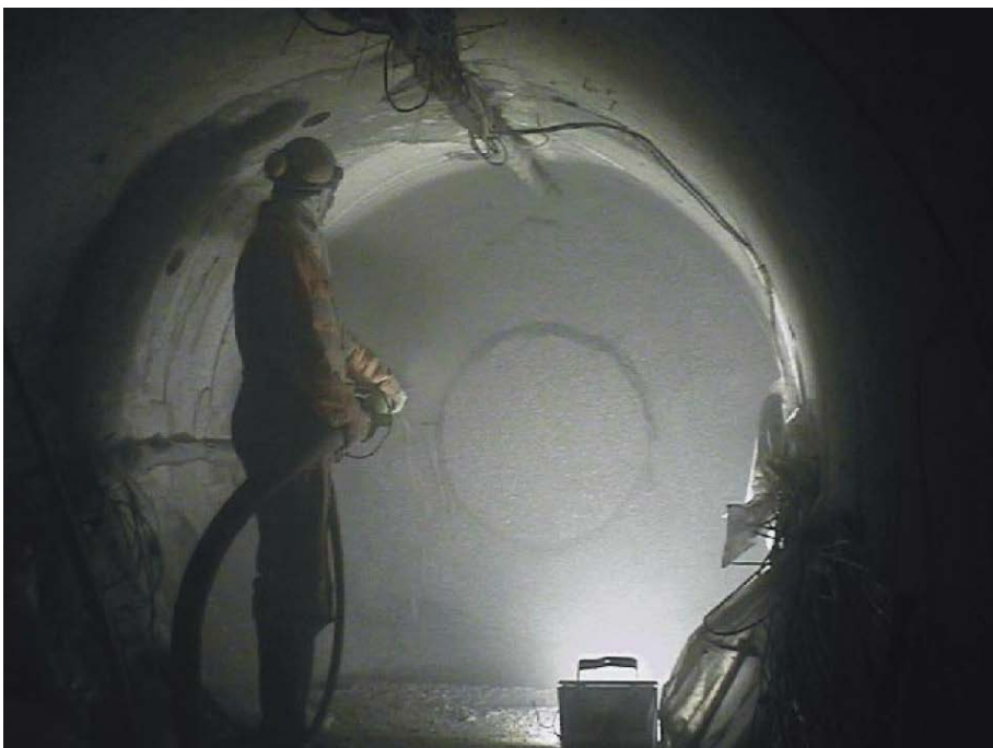
Figure A-43. Shotcreting of the first layer onto the bentonite front (Bárcena et al. 2003).
