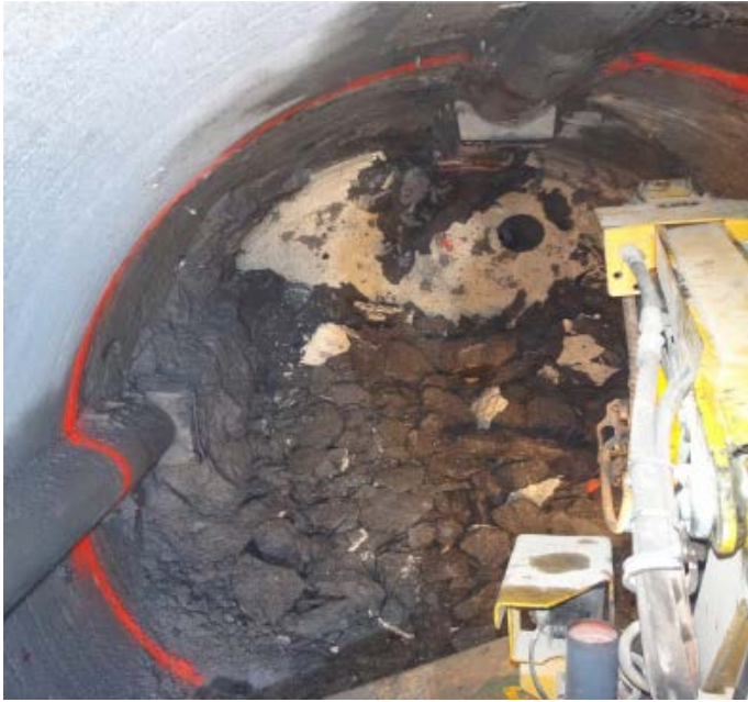
Figure B-4. Marking of plug face on the gallery (red) and partial view of the autonomous robot. Some debris were left on the bottom of the tunnel to facilitate the robot movement (García-Siñeriz et al. 2016).
