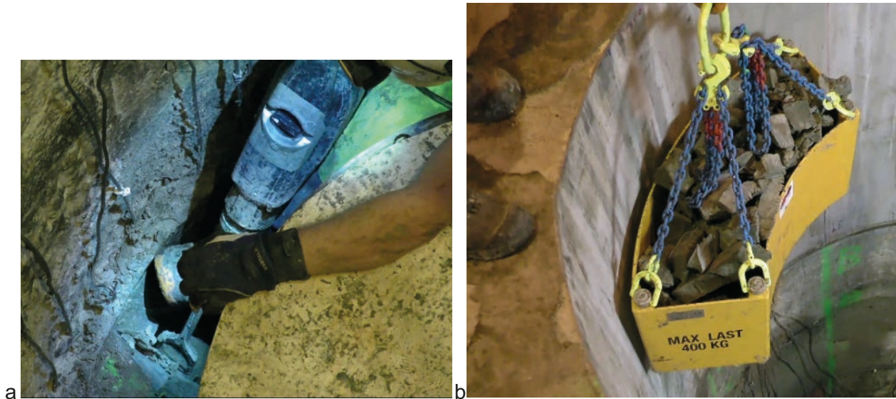
Figure 15-22. Removal of the buffer. a) Jack hammers were necessary to break the bentonite; b) Removed material was craned to the surface for disposal.
