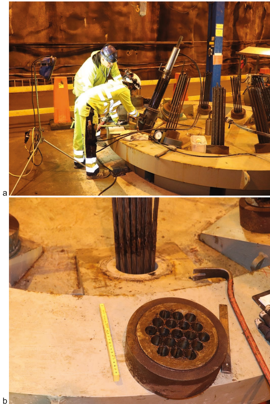
Figure 15-17. Removal of the anchor system. a) Loosening the anchor cable stop using a hydraulic tool; b) Anchor cable stop after removal.
