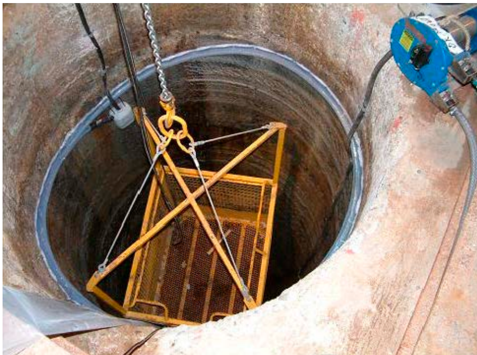
Figure 2-6. Deposition hole DA3147G01 with the circular drain and small plastic container (greyish) used to collect inflowing water.
