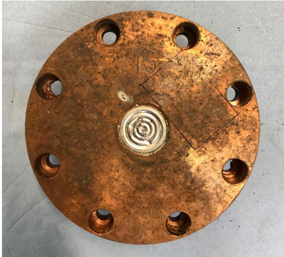
Figure 3-2. Overview of filter housing PC901 and the area of which sample coupons for analysis were to be taken, marked on the filter housing with a black rectangle.
