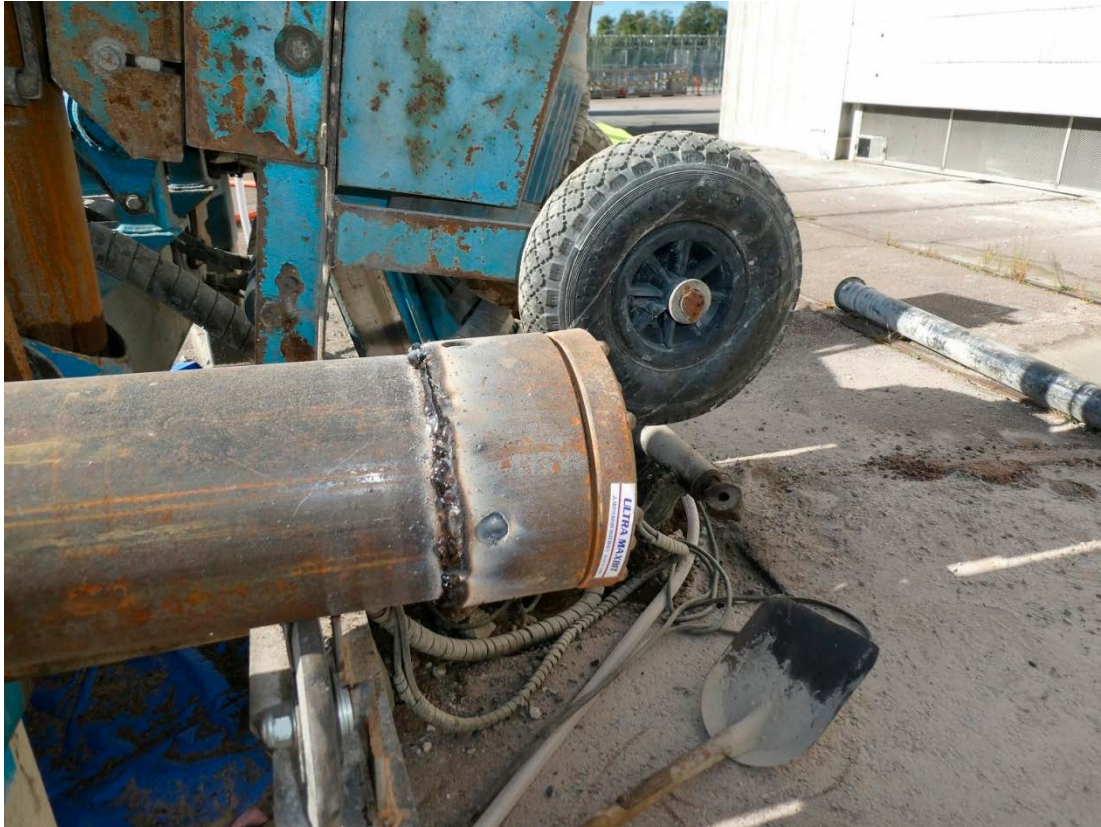
Figure 4-1. The Ultra Maxibit system applied on a standard casing was used fro pre-drilling through overburden in KFM25, KFM26, and KFM27.
