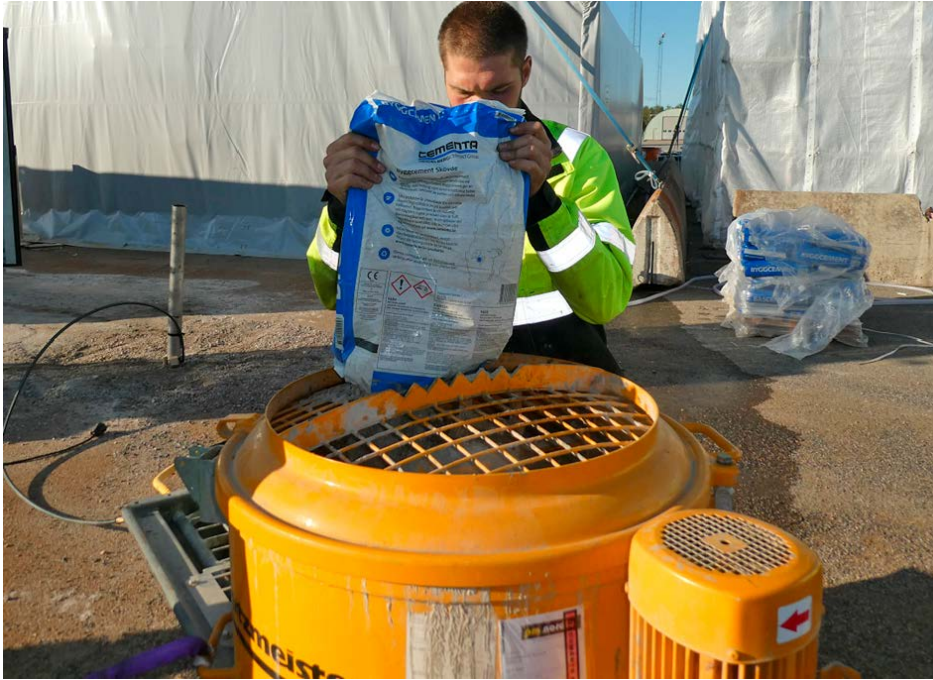
Figure 3-3. Grouting of the gap between the outer and inner casing was performed by pumping the cement through a hose from the bottom of the borehole.
