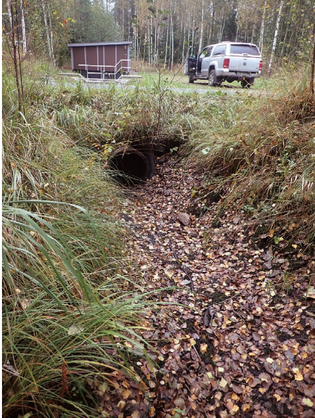
Figure 3-3. Dry conditions at PFM000068 in October 2020.
