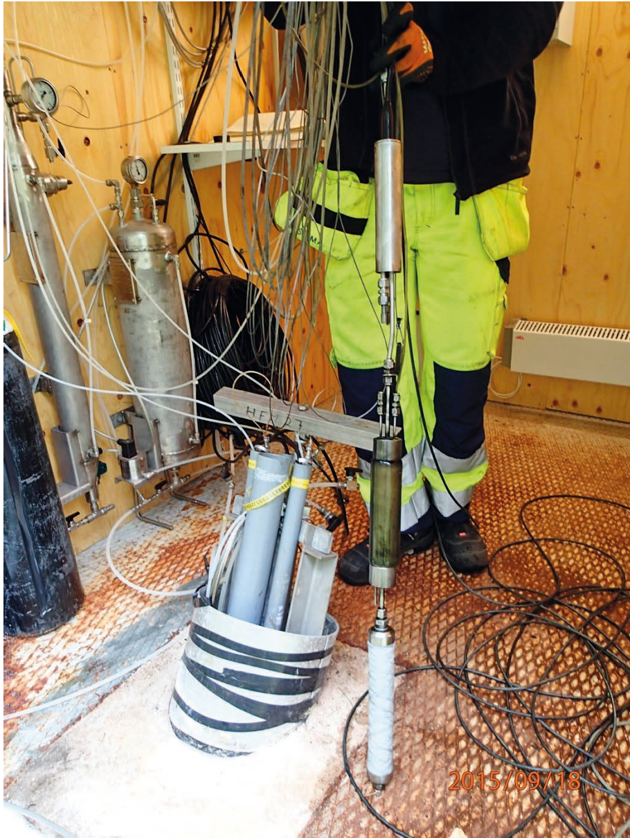
Figure 2-3. The pumping equipment (GEOPUMP UV-45) used for pumping in wide standpipes. The equipment consists of a filter and a pump connected to the mini-packer. The small diameter plastic hose is used for expanding the packer and the plastic hose connected to the pump is the pumping hose (enclosed picture right lower corner).
