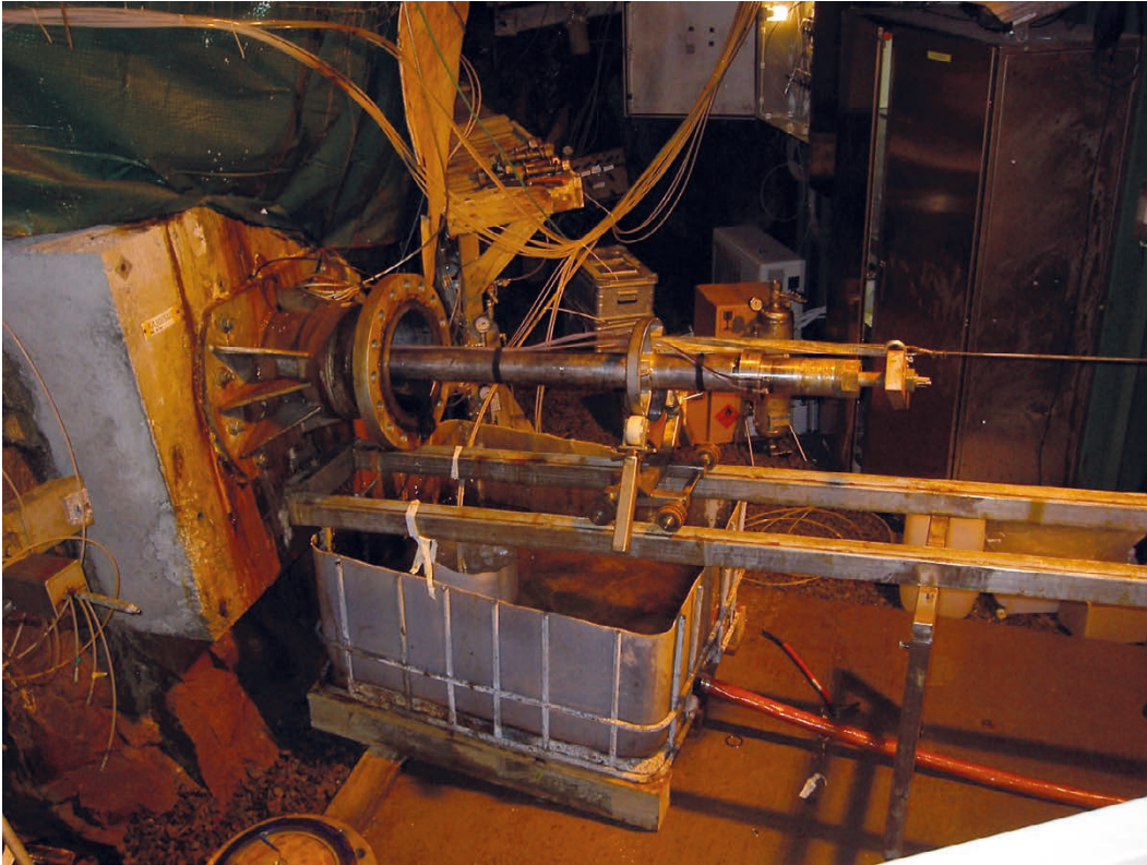
Figure A6-3. Lid at borehole collar removed and packer system is hauled out of borehole KA3065A03. Container beneath borehole collar, where water was sampled and monitored for \gamma -radiation, is also shown in the photo.
