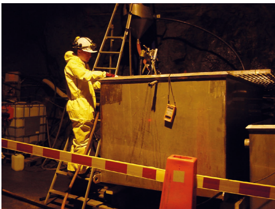
Figure A7-2. Check of installation at sedimentation container 1. Low dose scintillation meter attached to container wall for continuous measurement of radioactivity in the backwashing water.
