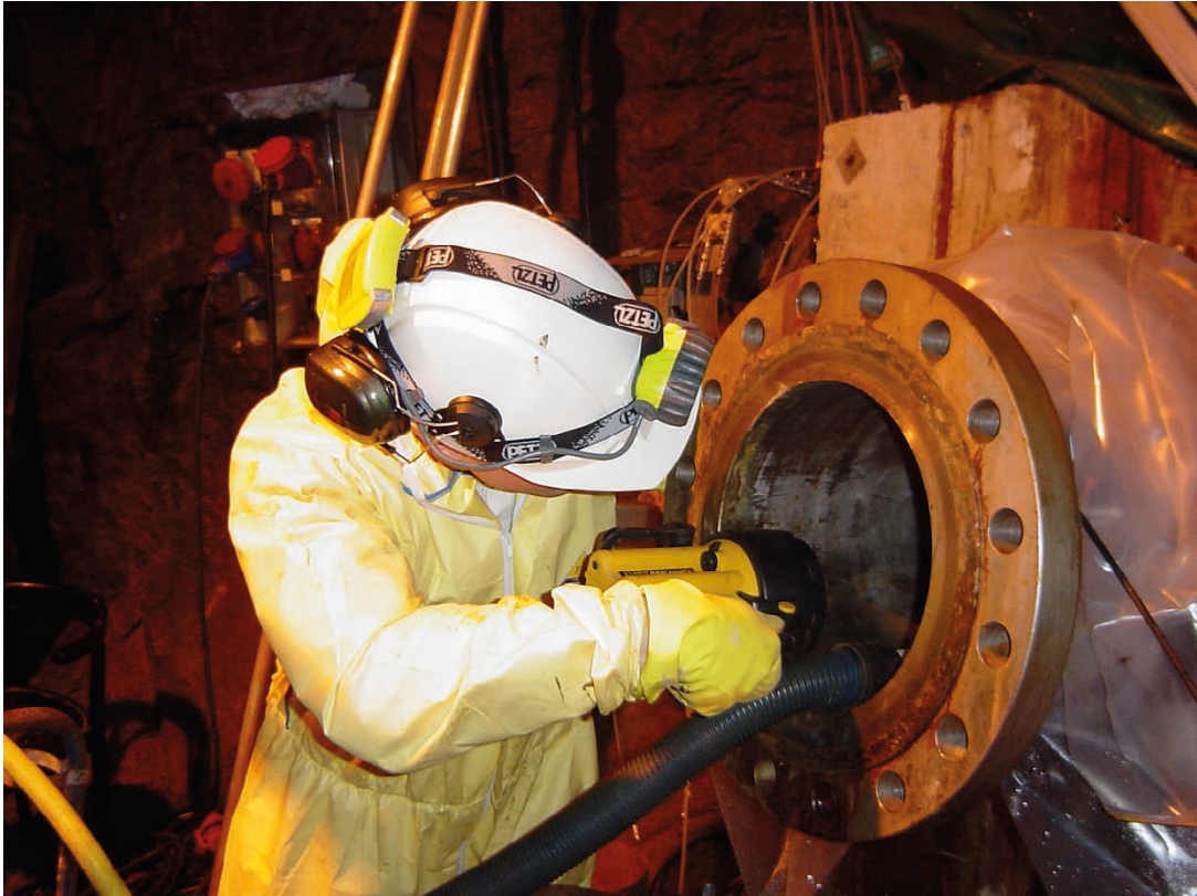
Figure A7-16. Borehole is drained by suction pump and inspected before start of drill phase 2.
