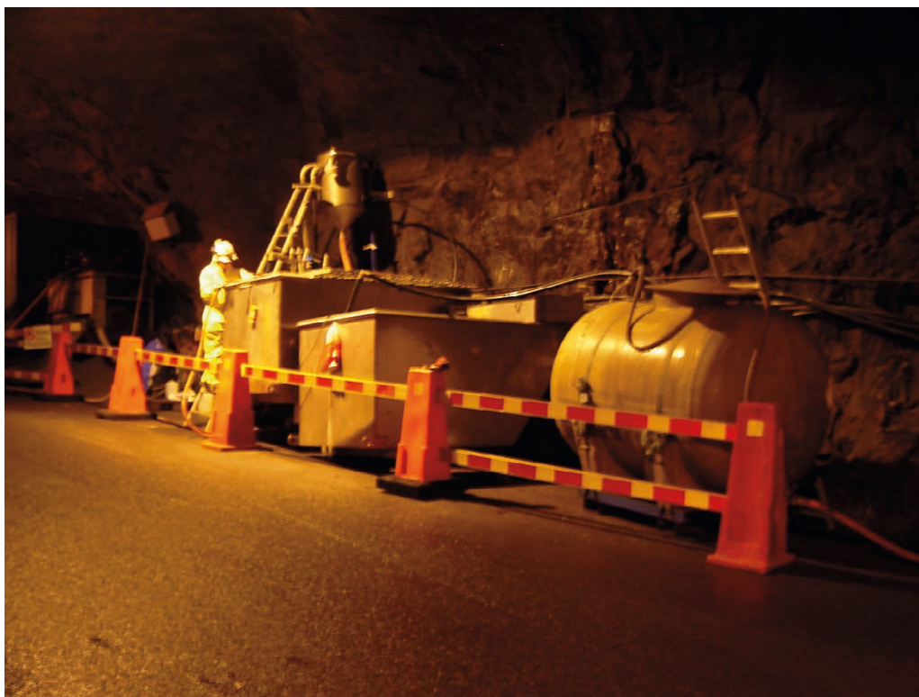
Figure A7-1. System for handling backwashing water. Degasser (cyclone) on top of sedimentation container 1.
