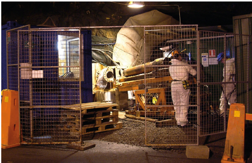
Figure 2-11. Drilling machine (Onram 1000) with 300 mm diameter drillbit and core barrel are checked prior to over-core drilling borehole KA3065A03.
