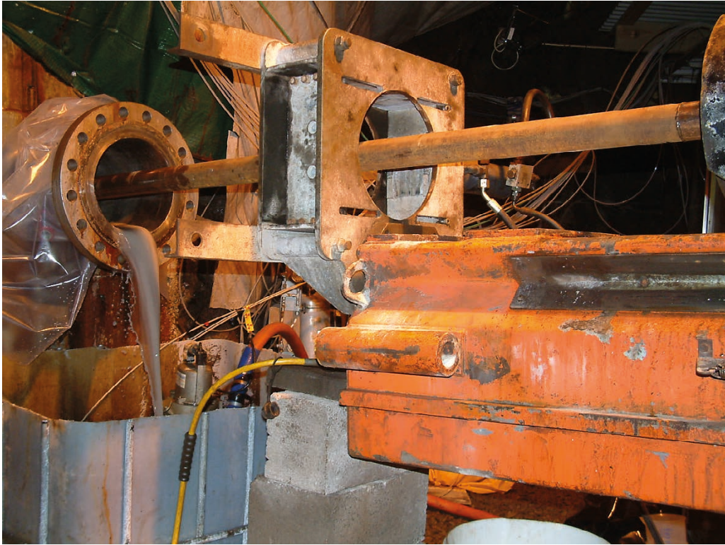
Figure A7-5. Ongoing over-core drilling. Backwashing water with drilling debris flowing into container beneath borehole collar.
