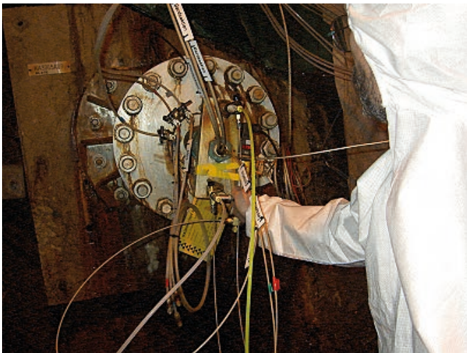
Figure 2-5. The yellow coloured (EpoDye) epoxy resin being injected at the KA3065A03 borehole collar.
