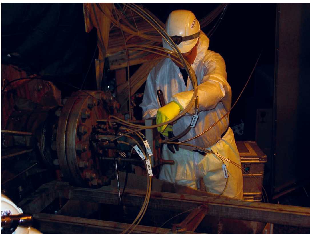
Figure A6-2. Tubes and fittings being disconnected before the lid at KA3065A03 borehole collar is removed.
