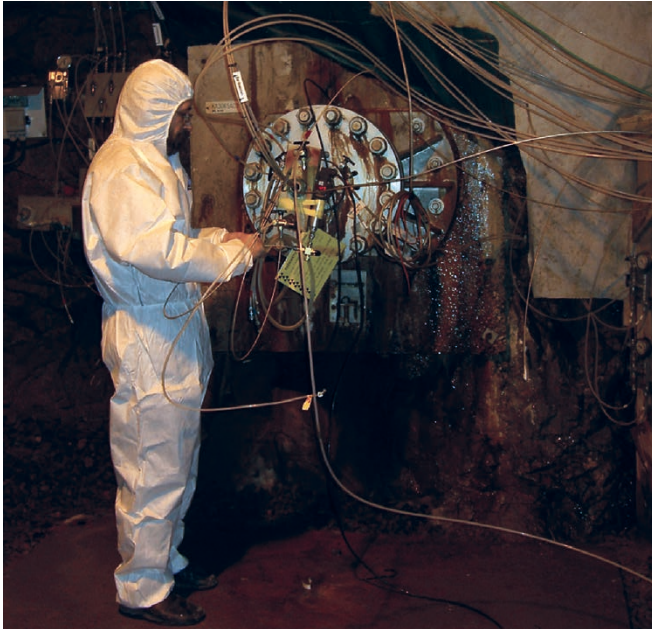
Figure 2-4. Cutting circulation tubes under pressure at initial phase of epoxy resin injection.
