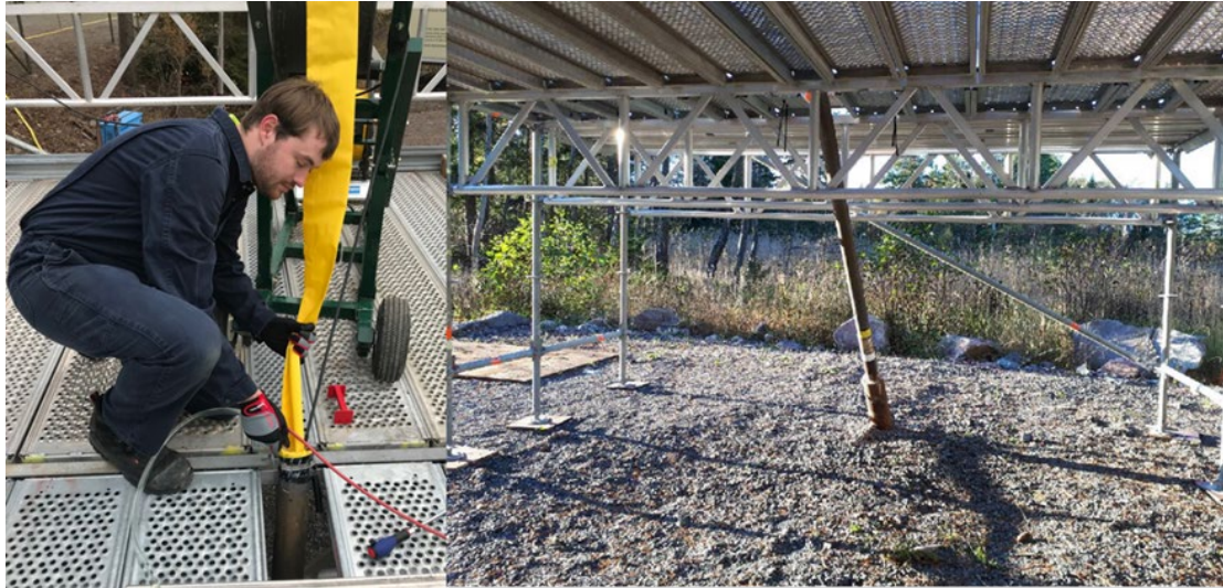
Figure 5-1. FLUTE installation (left) and KFM16 head extension with the platform (right).
