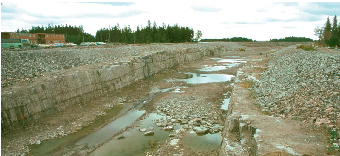
Figure 1-11. Picture from the construction of the 13 m deep and more than 1 km long canal between the Baltic Sea and the nuclear power reactors at Forsmark. Horizontal sheet joints are encountered along the entire excavation. The sheet joints follow the undulations of the bedrock surface (Photo: G. Hansson).
