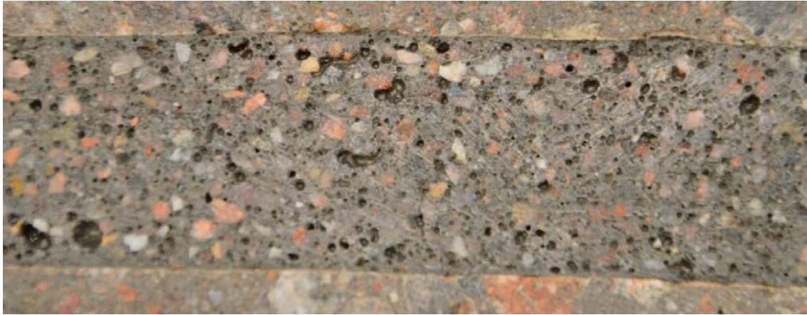
Figure 3-15. Cross section of a grouted hole. Note the presence of a large number of voids in the grout.
