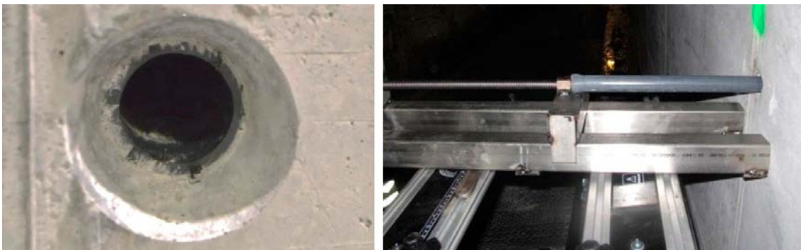
Figure 3-14. The images show the protective tube left in the concrete (left image) and during extraction.
