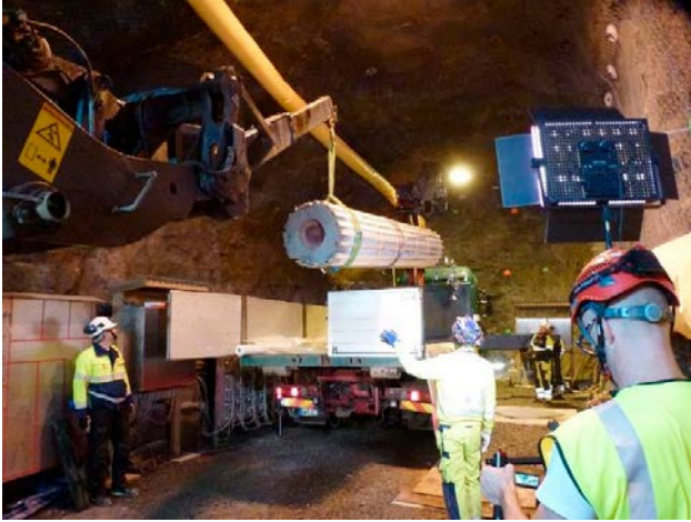
Figure 3-37. The entire test parcels, including rock-cover, were being placed on a lorry for transport to the ground surface.
