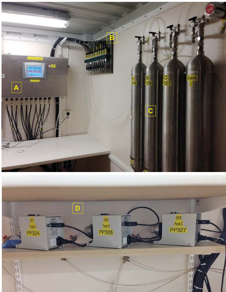
Figure 2-2. Parts of TDE injection container in the REPRO niche, containing equipment such as data acquisition (A), pressure transducers (B), pressure regulation vessels (C), and circulation pumps (D).
