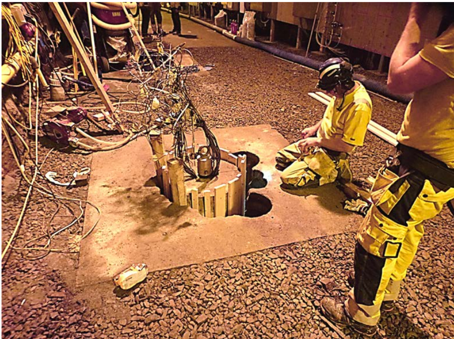
Figure 5-1. The released test parcel ready to lift (A3). Note the surrounding slot made by overlapping percussion drilled holes and the larger core drilled holes.
