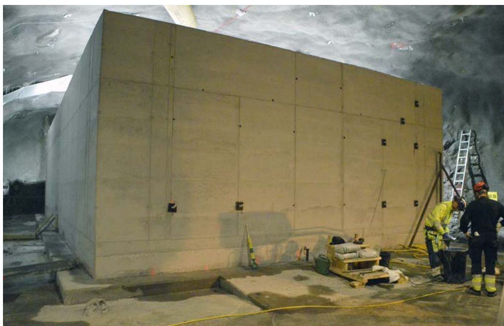
Figure 9-1. Some of the holes used in the concept test have been covered with a wooden board with a hole provided with a plastic hose for injection of the grout.
