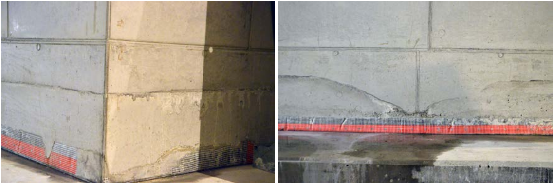
Figure 8-14. Joint between the base plate and wall in an area with the correct casting of the base slab (left) and in an area with poor filling in this section of the base slab.
