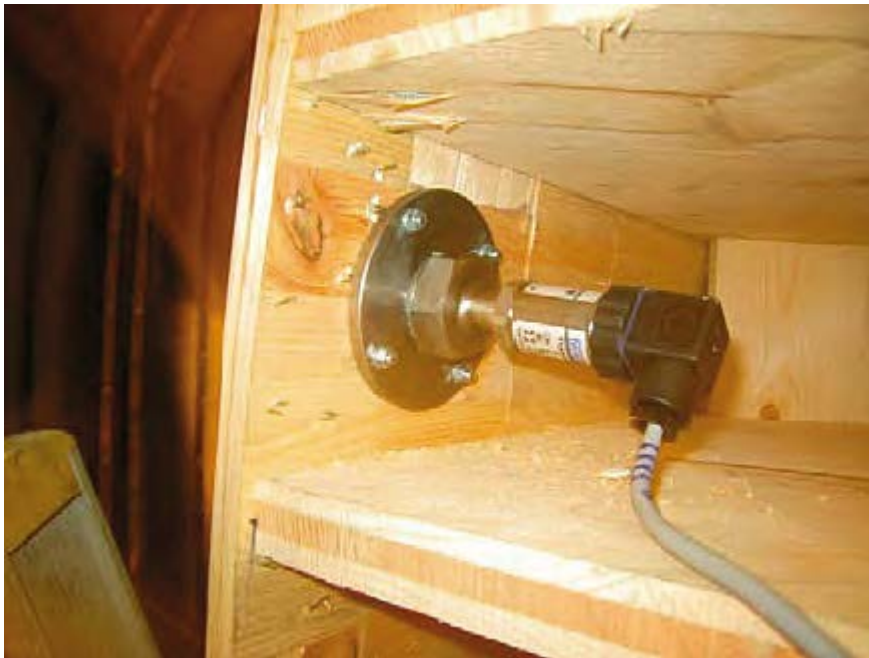
Figure 3-8. A pressure sensor installed in the formwork of the Dome Plug at Äspö. From Grahm et al. (2015).
