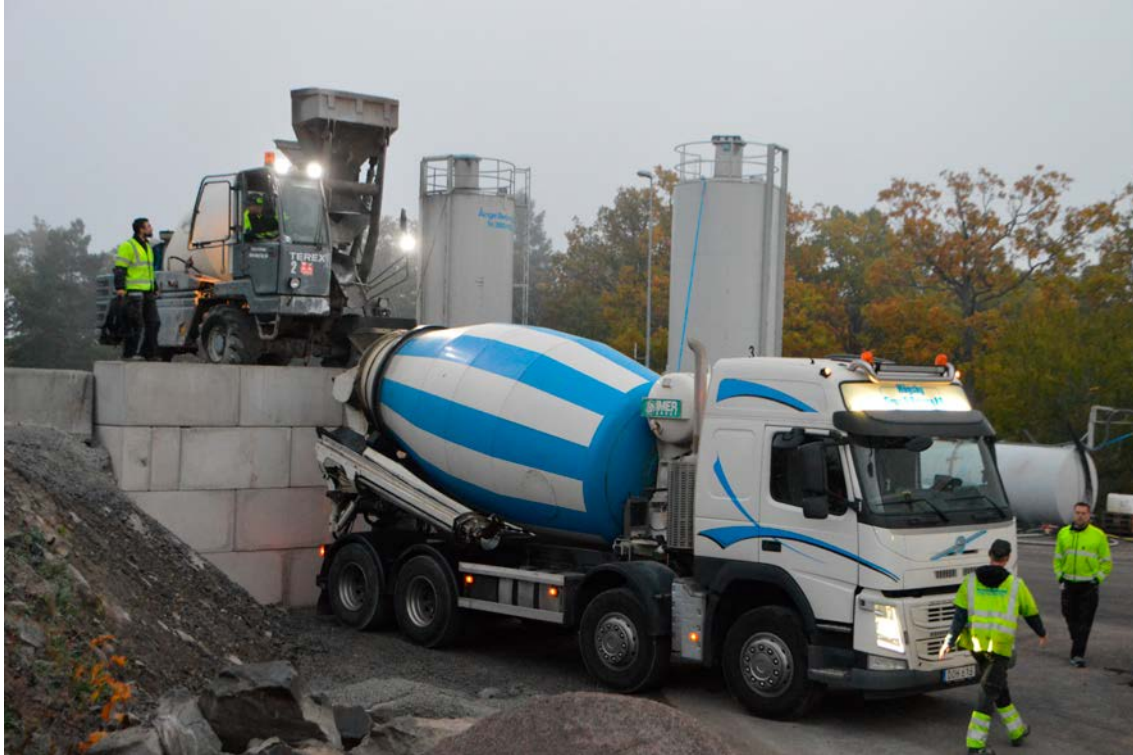
Figure 5-14. The truck mixer is positioned for pouring of the concrete into the transport truck.
