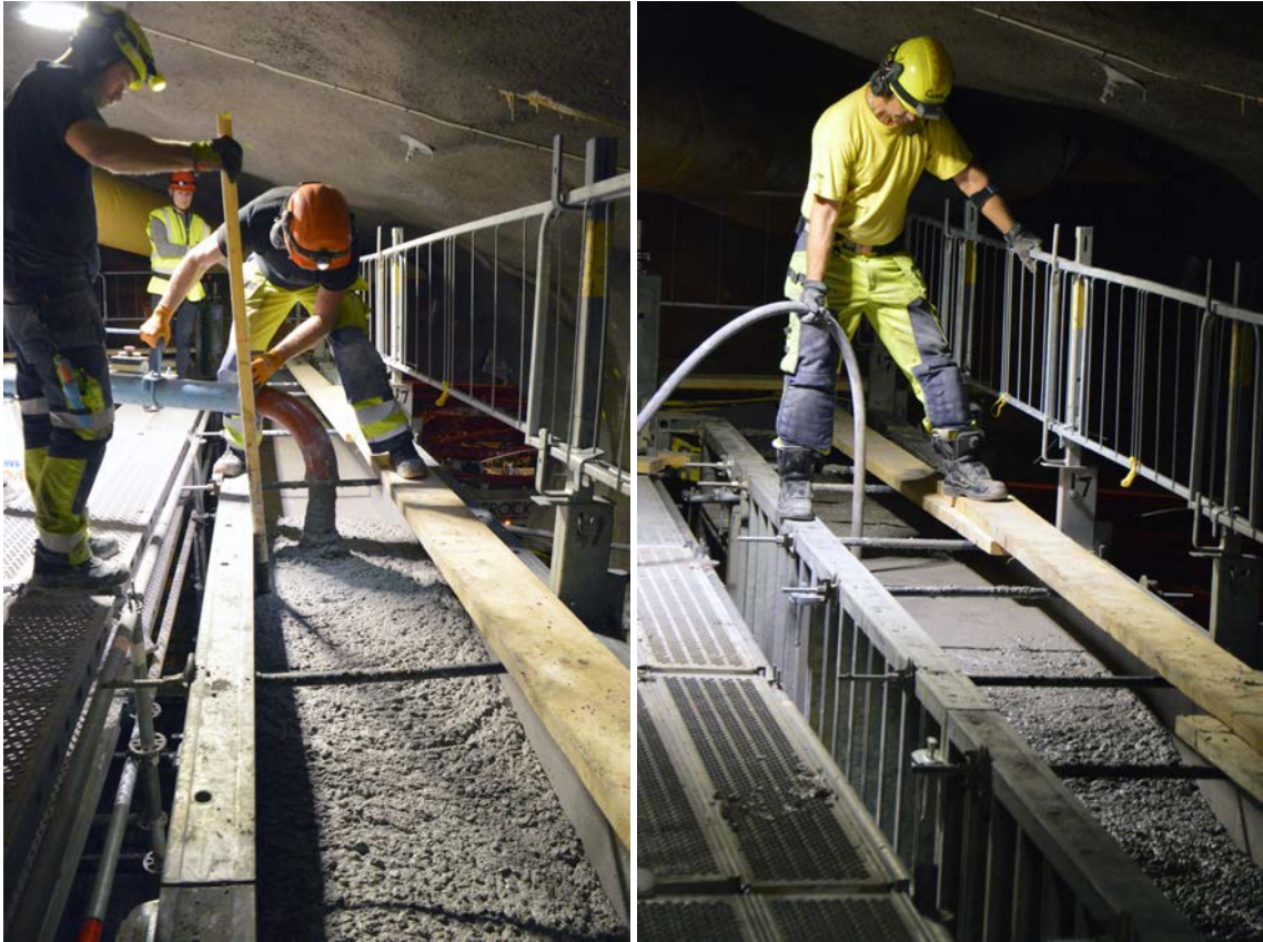
Figure 8-9. Placement of the concrete and vibration in the upper part of the wall.
