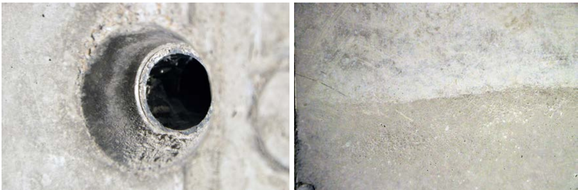
Figure 8-13. The picture on the left shows a protective tube for a tie rod and the one on the right shows a colour change in the wall caused by the use of concrete from 2 different trucks. In the right image, the contrast has been enhanced compared to the original image.
