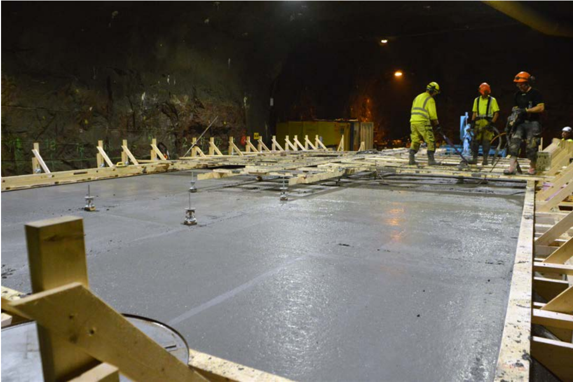
Figure 7-14. As casting proceeded, the footbridge was removed and the surface of the slab trowelled.
