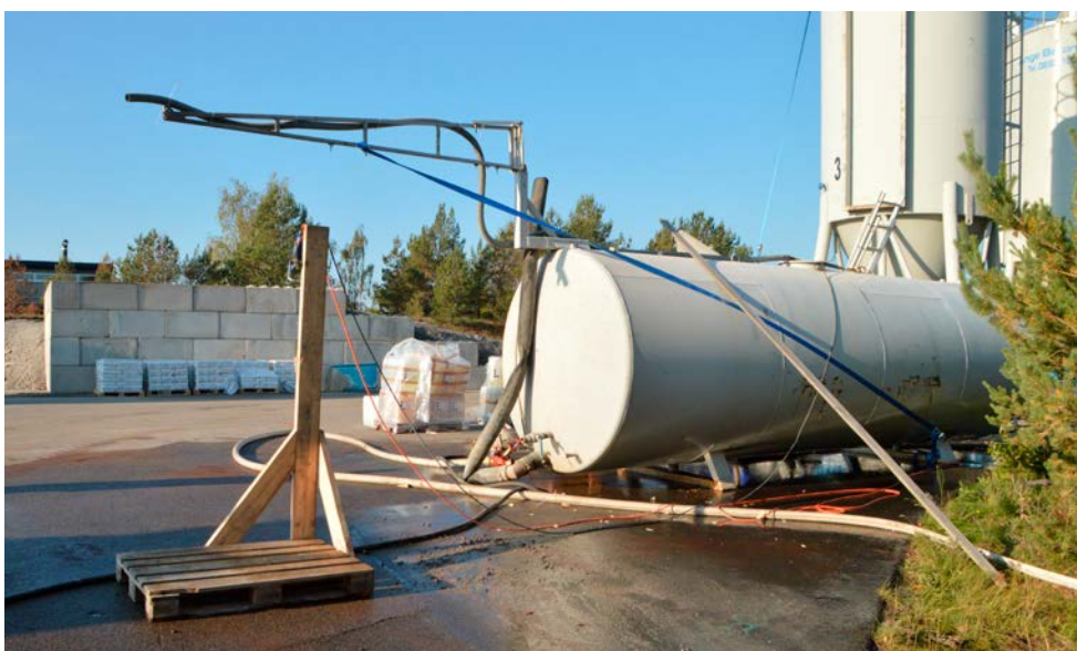
Figure 5-7. The water tank was placed near the silos. In the tank was a powerful pump for quick filling of the truck mixers which could be started and stopped by means of an electric switch attached to the post in the left part of the image.
