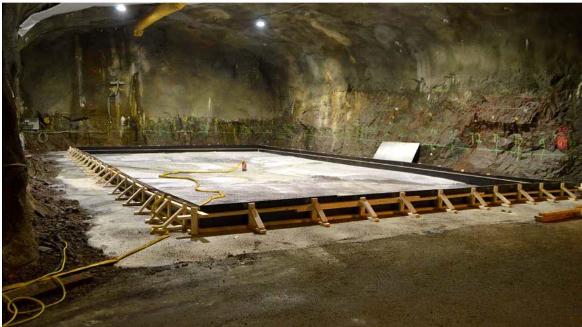
Figure 4-4. After filling of the largest pits also in the inner part of TAS08 and formwork construction for casting of the top layer.
