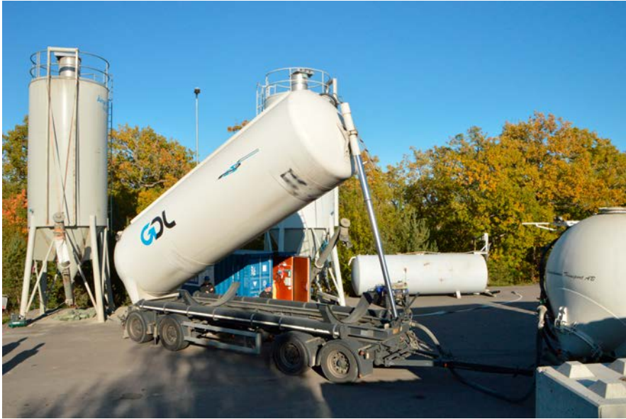
Figure 5-8. Filling of the cement silo.
