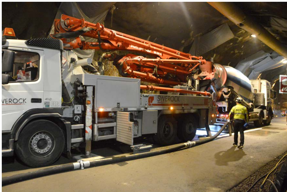
Figure 7-10. The concrete pump that was used during casting. It can be noted that the mast could not be used due to limited space. Instead, the hose was directly connected to the pump.
