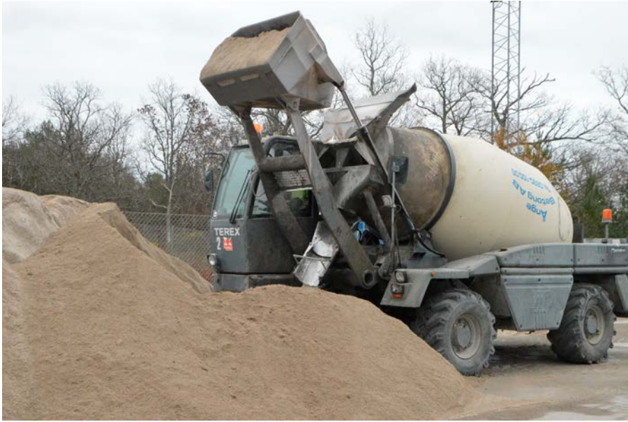
Figure 5-3. One of the two truck mixers during filling of gravel into the mixer.
