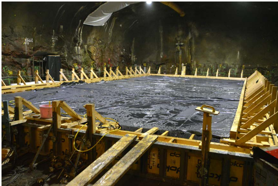
Figure 7-16. The base slab has been sprinkled with water and covered with a plastic sheet.
