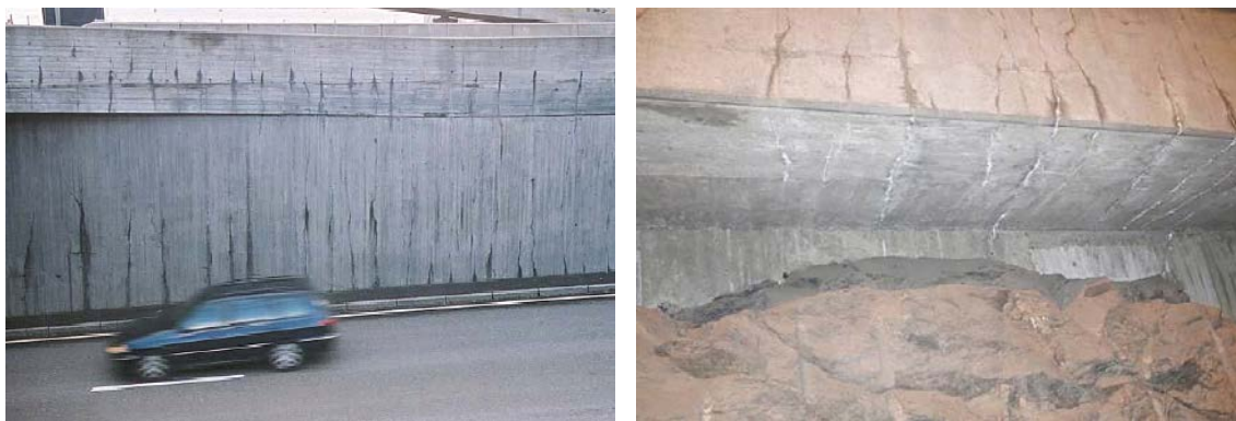
Figure C-1. Early age cracks in retaining walls, left picture: Anders Hösthagen, BOSTEK, right picture: Jonatan Paulsson-Tralla, BOSTEK.
