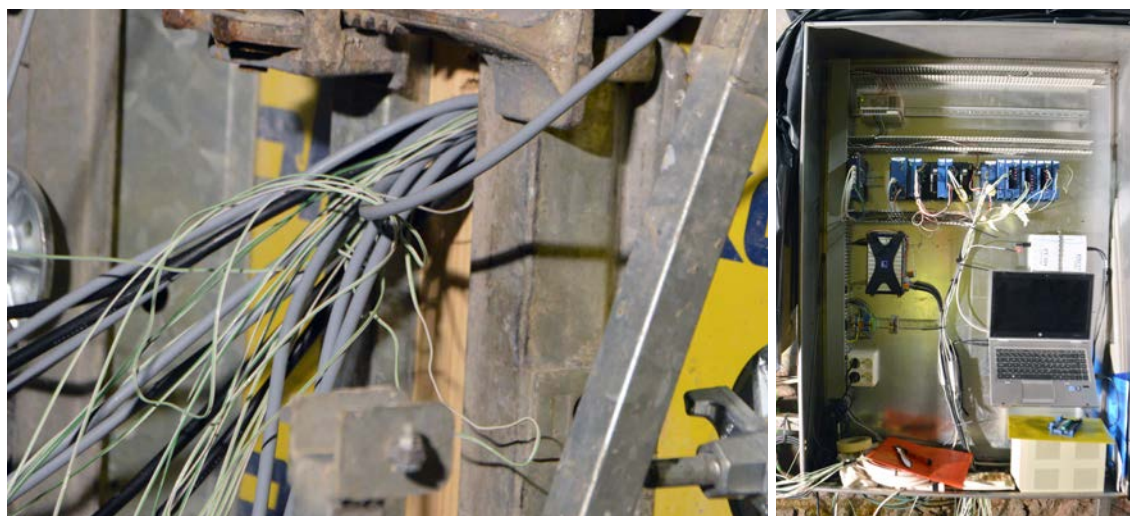
Figure 7-8. The cables were collected into one bundle connected to the control cabinet through a hole in the formwork.
