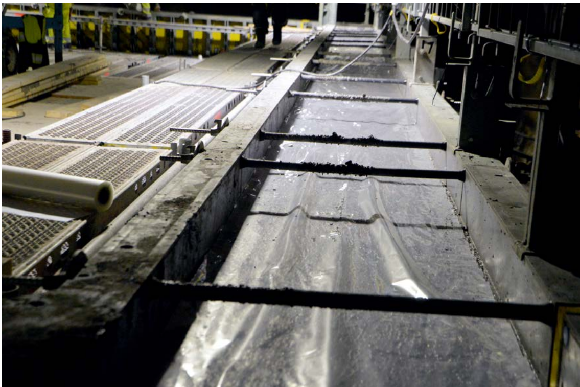
Figure 8-11. The top surface of the concrete has been covered with a plastic foil.
