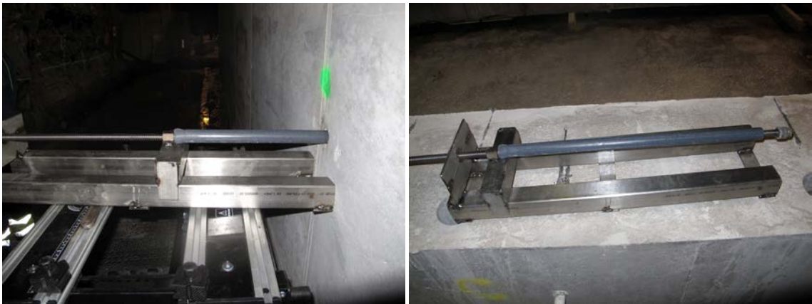
Figure 9-14. The extraction tool has been mounted against the concrete wall (left image) and the tube extracted (right image).
