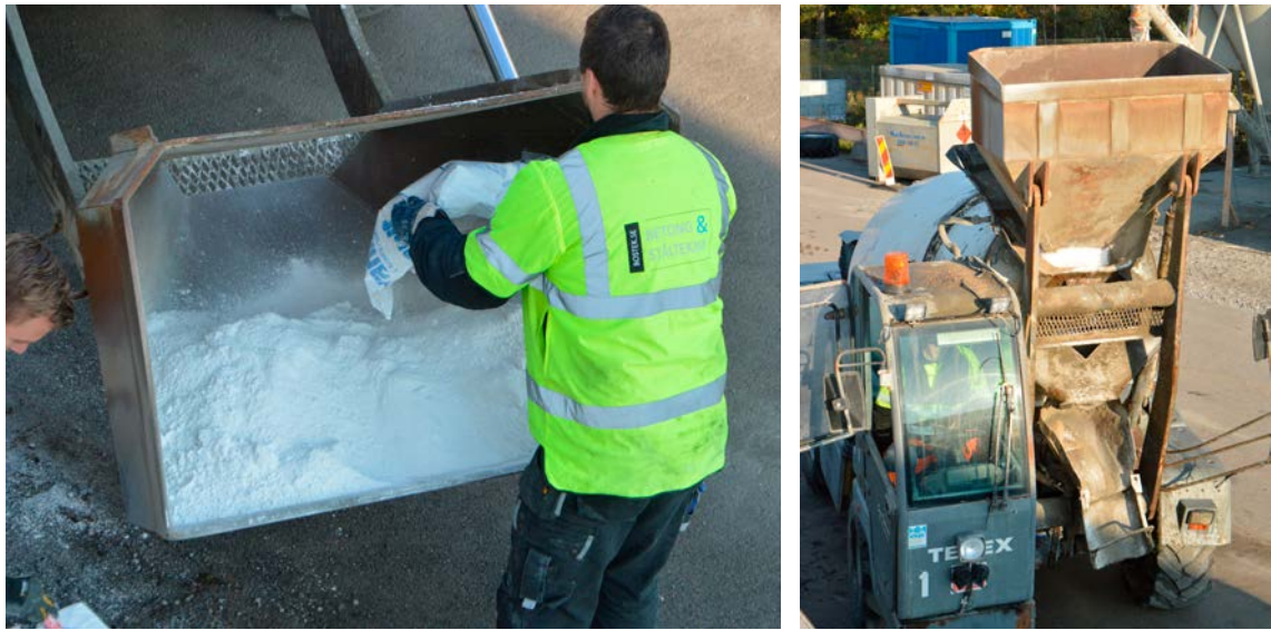
Figure 5-12. Filling the loading bucket of the truck mixer with Myanit 10 and feeding of the mixer.
