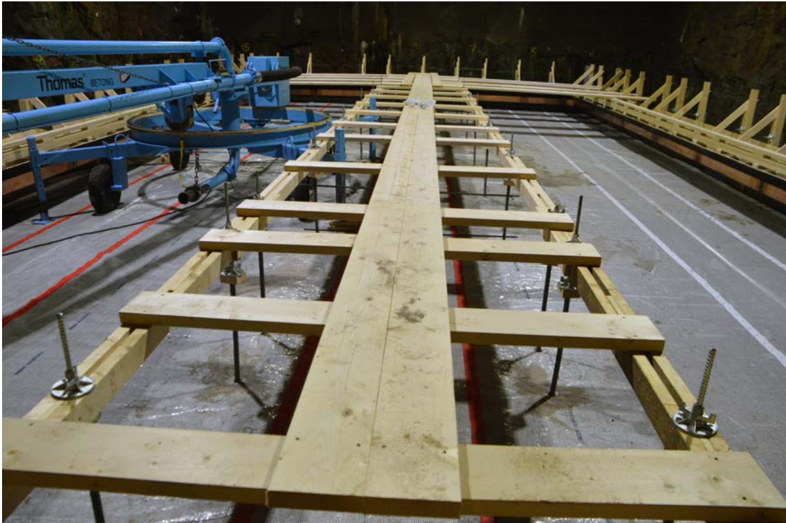
Figure 7-4. The central footbridge of the platform used during casting of the base slab.
