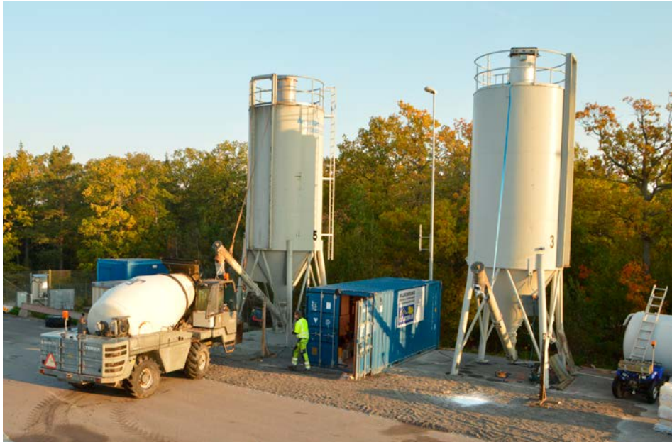
Figure 5-6. The silos have been erected and assembled and a layer of gravel has been laid out for protection of the asphalt surface.
