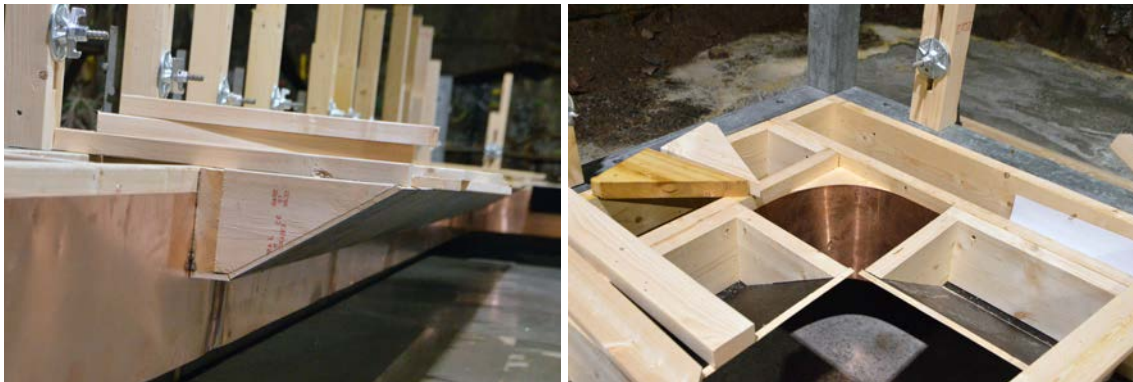
Figure 7-3. Details of the on-site built formwork for the recess, also showing details on how the joint seal was mounted in the formwork.
