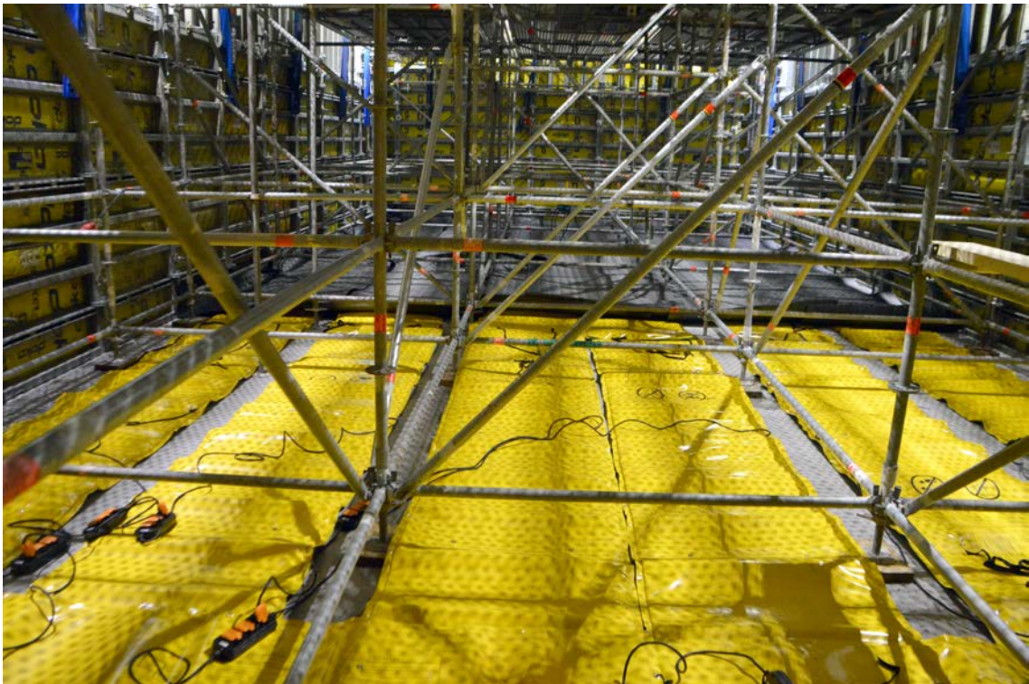
Figure 8-4. Heating mats have been placed over the entire base slab with insulation covering the inner parts.
