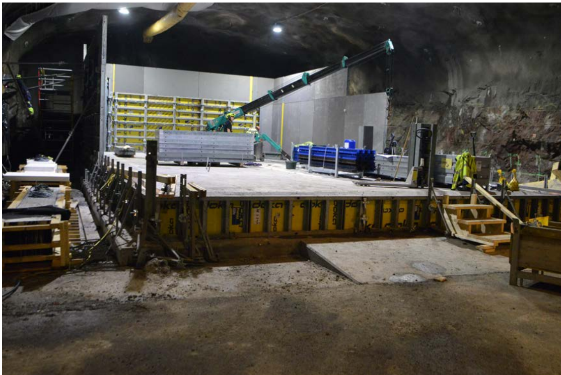
Figure 7-17. The base slab after partial disassembling of the formwork and start of erection of formwork to the walls.
