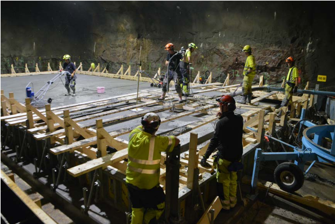
Figure 7-15. Towards the end of the casting, several activities were carried out simultaneously. While casting was still in progress in the outer parts, disassembling of the footbridge and trowelling was carried out in the inner parts.
