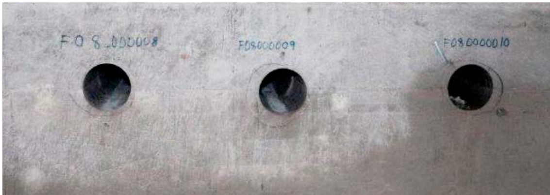
Figure 8-18. Holes after extraction of cores from the joint between the base slab and one of the walls.
