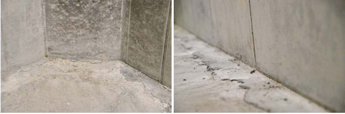
Figure 8-15. Visual appearance of the joint on the inside of the concrete caisson.
