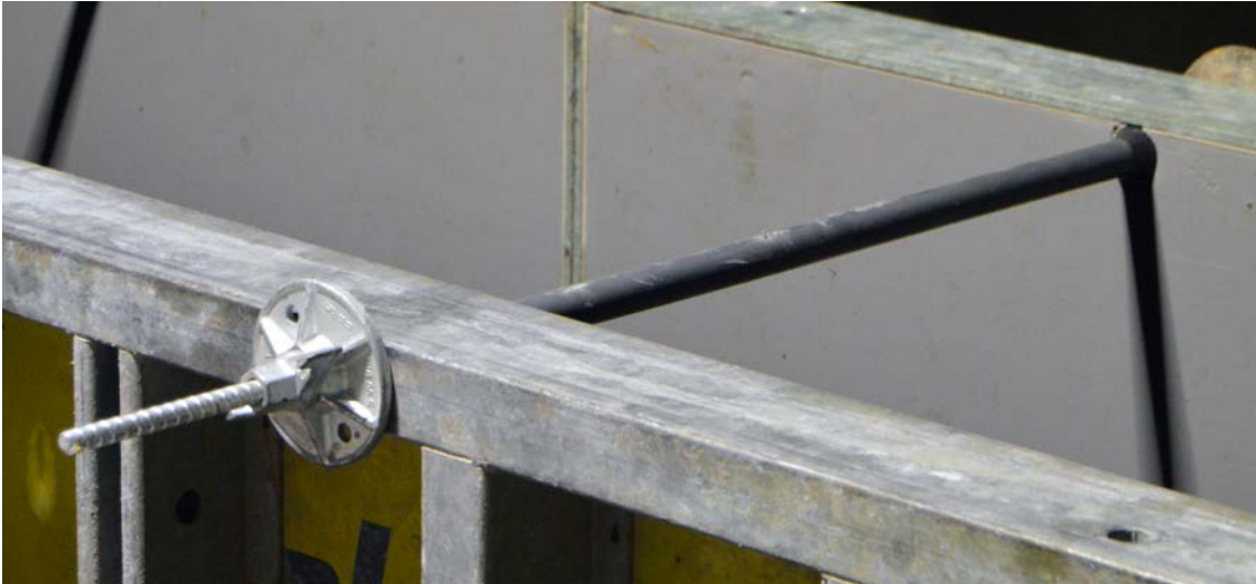
Figure 8-2. A tie rod which is protected by a plastic tube in the upper part of the formwork.
