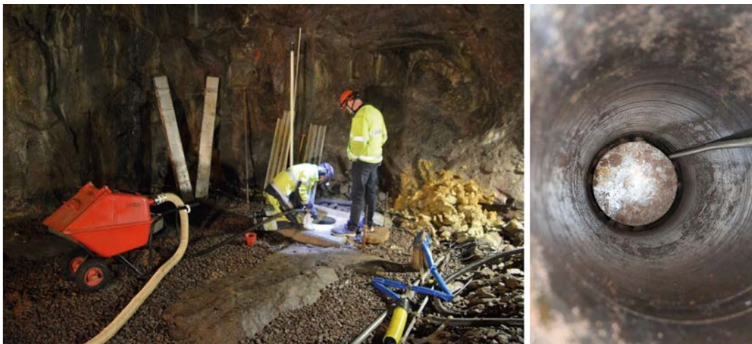
Figure 2-3. Cleansing of the sand filled slit between the concrete cylinders and the wall of the installation hole.
