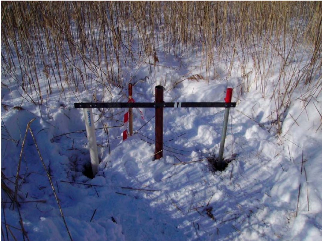
Figure 3-9. Example of anchoring by means of mutually supporting pipes connected by iron bars (wells SFM0091–93; Werner et al. 2006).
