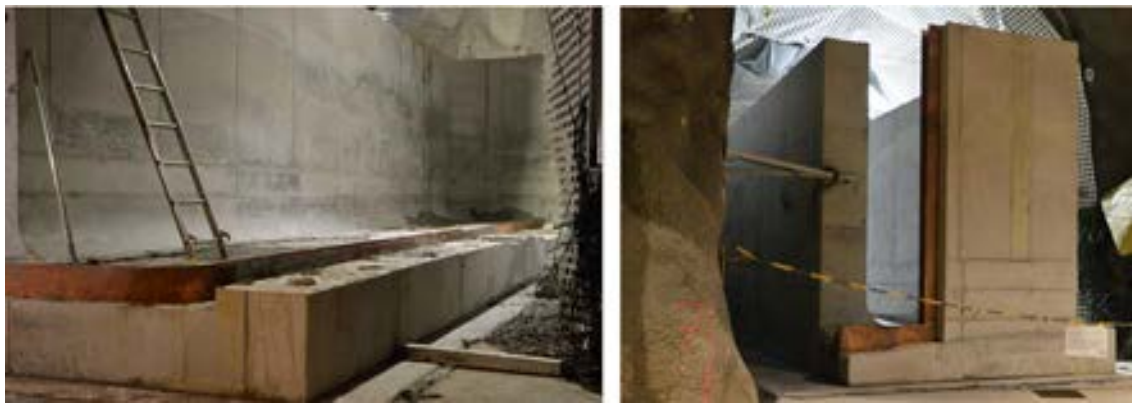
Figure 10-3. Caisson section 1 including base slab and L-shaped wall (left), and caisson section 2 including L-shaped wall, which was built on the base slab of section 1.
