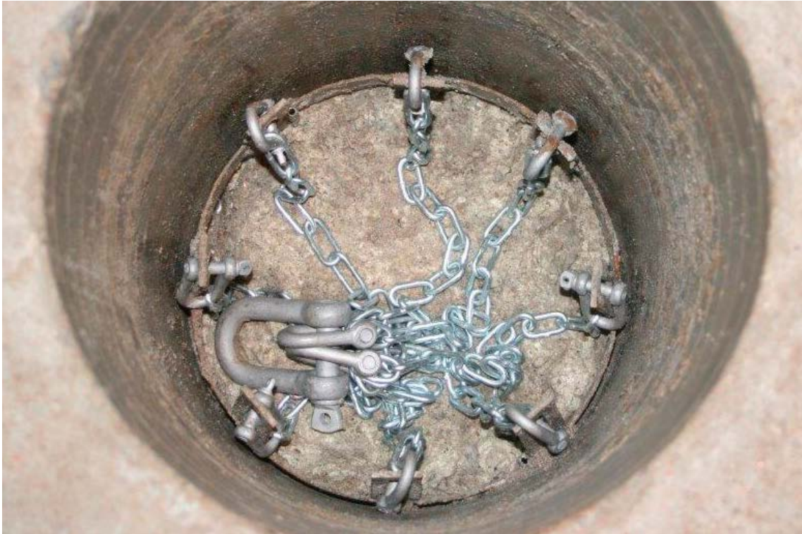
Figure 2-4. Lifting eyelets have been mounted in the flat irons before the first lifting attempt.
