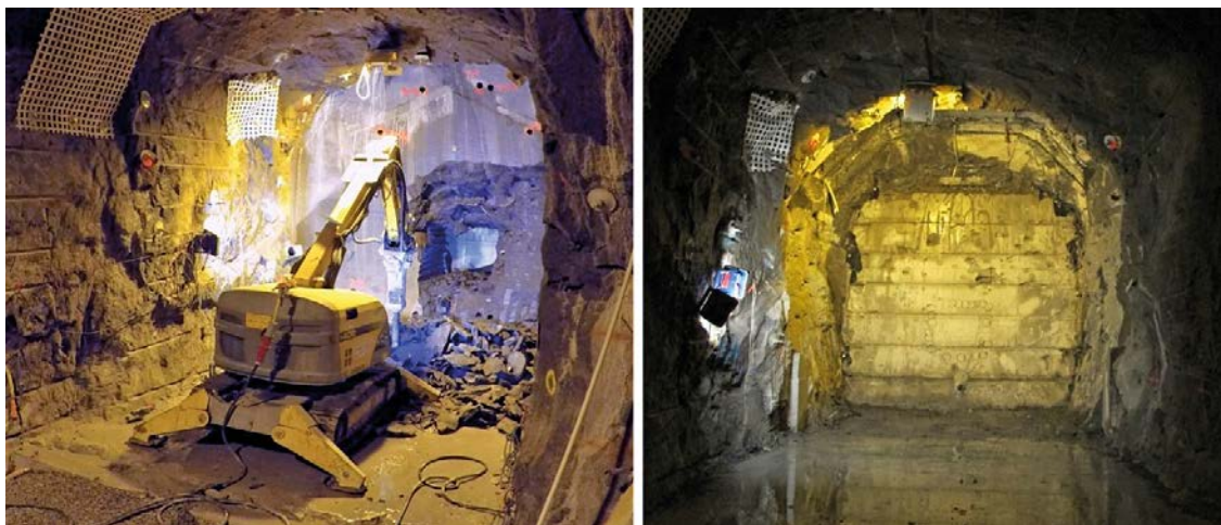
Figure 3-5. Machine for breaching (left) and result after removal of the concrete dome (right).
