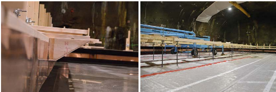
Figure 3-17. Images showing how the joint seals were fixed in the part of the form work shaping the joint, left image, and the plastic sheet used to reduce adhesion between the foundation and the base slab of the caisson.
