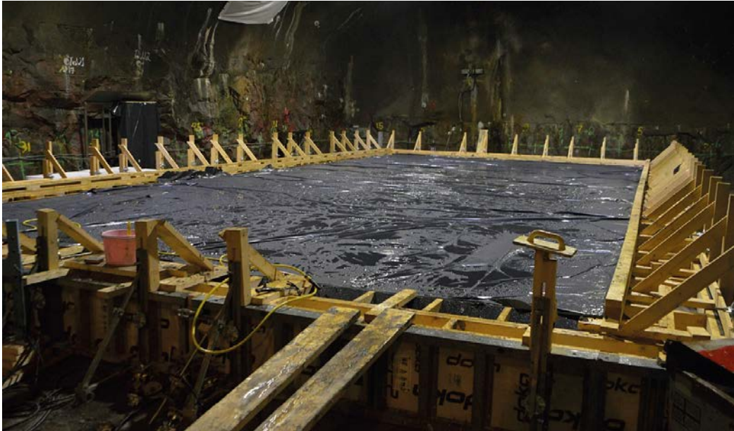
Figure 3-19. Casting complete and the base slab sprinkled with water and covered with a plastic sheet.
