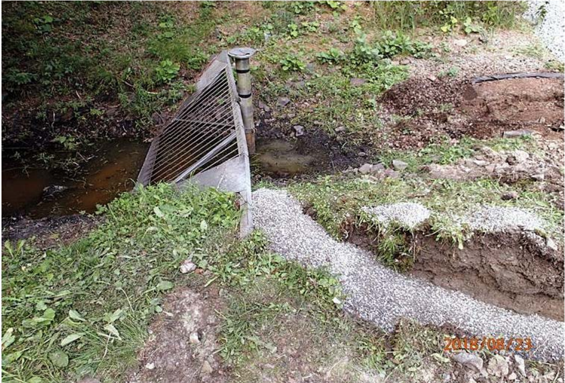
Figure 2-5. Upstream grating and tube hosting the EC and temperature sensor. As can be seen in the picture, the tube is mounted to the grating and communicates with the stream water not only through the tube screen but also through the open tube bottom.
