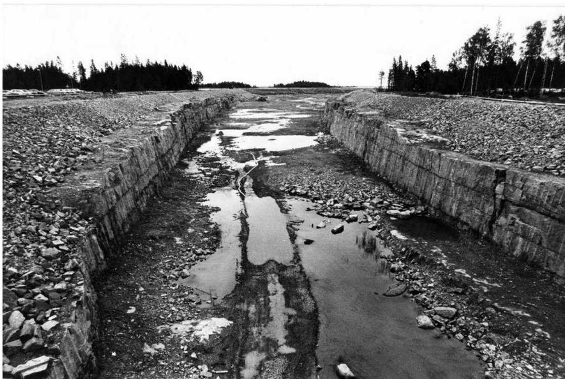
Figure 2-26. Horizontal fractures along the excavation made during the construction of the ca. 8 m deep and more than 1 km long canal at present sea level between the nuclear power plant at Forsmark and the Öregrundsgrepen. The section is located in the north-western part of the Forsmark tectonic lens (Figure 3-3); outcrops 0.2–0.5 km to the SE lack extensive sheeting. Photo: A. Carlsson.
