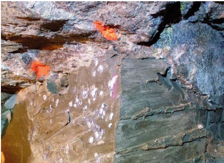
Figure 4-4. Photo taken during the excavation of the former pellet filled slot at the ceiling. The bentonite has swelled and is everywhere in good contact with the rock surface.
