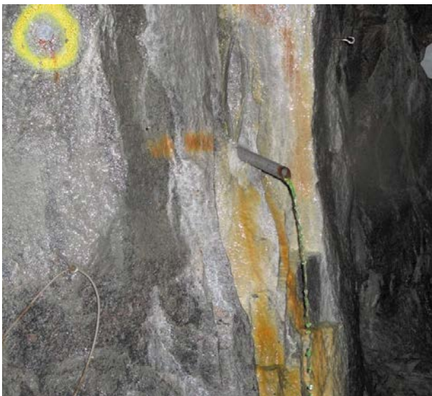
Figure 3-16. The water from the rock corner, see no.5 in Figure 3-13 is collected into a tube. The water is clearly colored by the uranine content.
