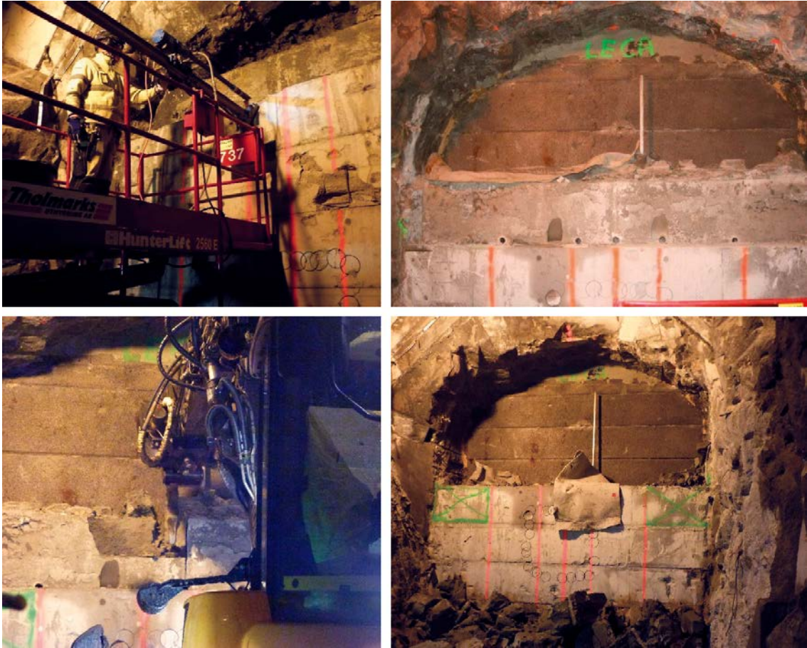
Figure 4-3. Upper left: A scissor platform was used during sampling of the bentonite. Upper right: The exposed bentonite has been sampled. Lower left: A special “hook” was used to remove the remaining bentonite above the next concrete beam. Lower right: The main part of the bentonite has been removed, leaving the outer parts close to the rock wall for sampling.
