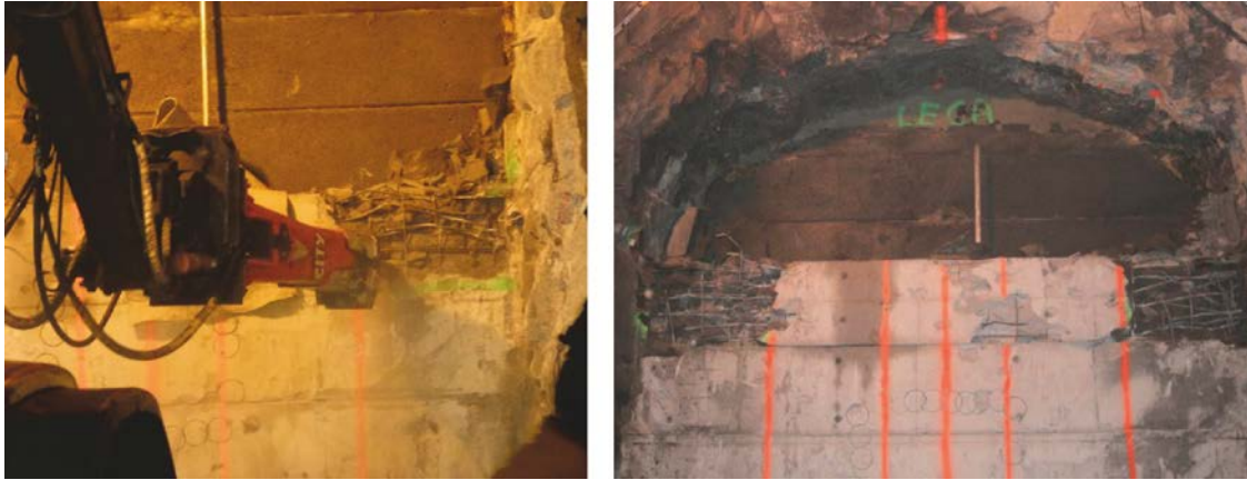
Figure 4-2. Left: A hydraulic hammer was used on both ends of each concrete beam to crush the concrete. Right: After crushing the concrete at both ends the steel anchoring to the rock was cut and the beam could then be lifted away by a large loading machine.
