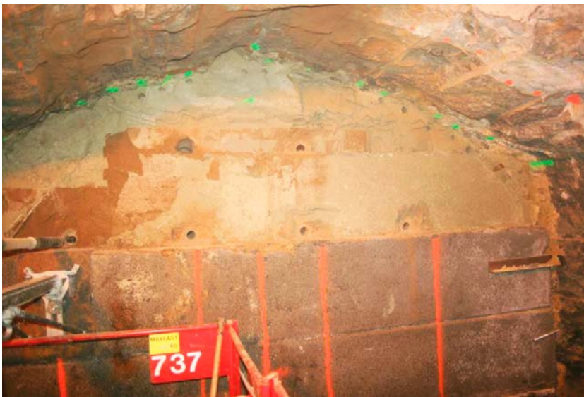
Figure 4-21. Photo showing the upper part of the backfill section after sampling. The core drilled holes in the central area can be seen and also the sampling of the backfill rock contour.
