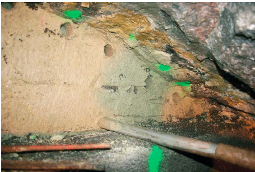
Figure 4-18. Photo showing a close-up of the contact between backfill bentonite and ceiling. The green dots shows the sampling points around the bentonite-rock contour at the ceiling.
