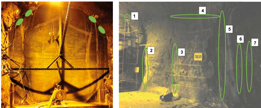
Figure 3-13. Left: Water leakages can mainly be detected at four positions in the interface between concrete and rock, see green marked areas on the photo. Right: Photo showing the areas where water leakages could be detected with the UV lamp. The photo is taken on the right side of the tunnel with the dome to the left in the photo.
