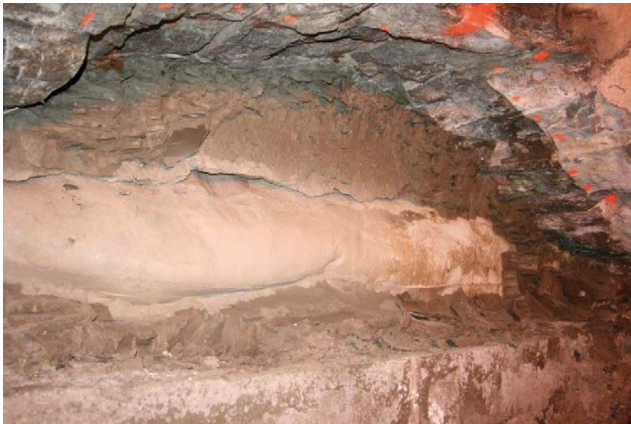
Figure 4-5. The photo shows the uppermost part of the bentonite seal and the geotextile separating the bentonite from the filter section. The geotextile is folded over the filter and bentonite pellets were blown into this gap during installation.
