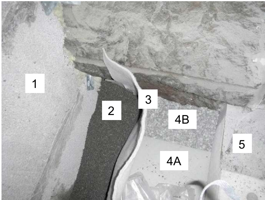
Figure 2-2. Photo taken during installation of the different components. From left: the LECA wall (1), the gravel filter (2), the geotextile (3), the bentonite seal consisting of block (4A) and pellets (4B) and the concrete beams (5).
