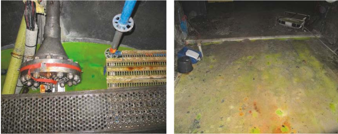
Figure 3-15. Left: The water standing in the weir in front of the plug has been colored by the uranine content in the leakage water. Right: Water has started to leak from the ceiling and are then dripping on the floor that is colored.
