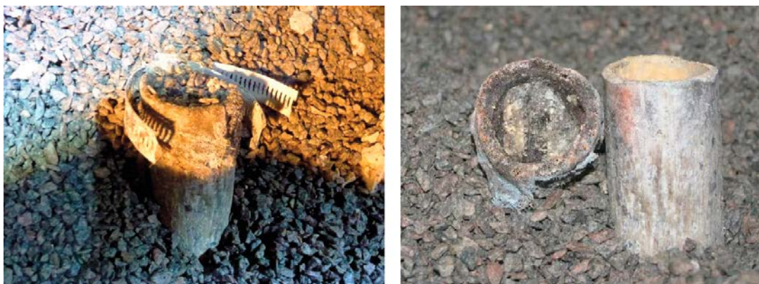
Figure 4-12. Left: Close-up of the upper de-airing tube with copper net and a broken hose clamp. Right: Close-up of the removed copper net placed beside the de-airing tube.
