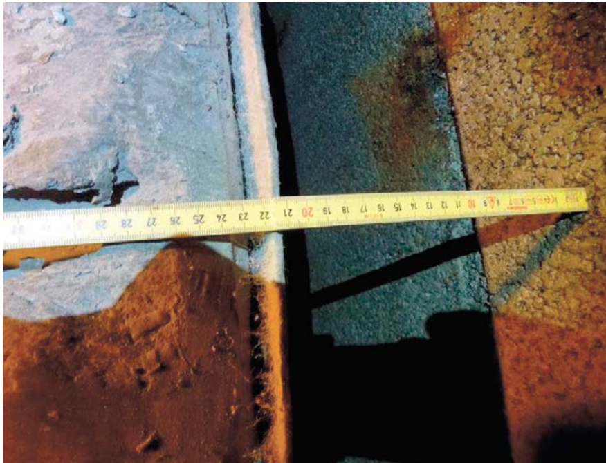
Figure 4-13. Measuring the filter section thickness at the upper level of concrete beam 5.
