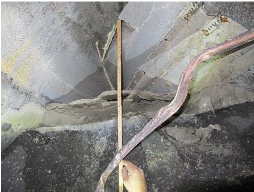
Figure 7-11. Measuring the height of the void, about 40 cm whereof 10 cm is filled with grout.
