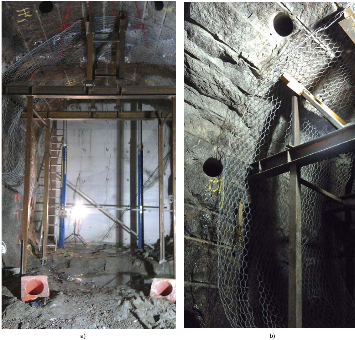
Figure 9-5. a) Erected safety scaffolding including a mesh to protect workers from falling rocks. b) Detail of the scaffolding with two of the Ø 250 mm boreholes for the wire-sawing are also visible. From Grahm et al. (2015) .
