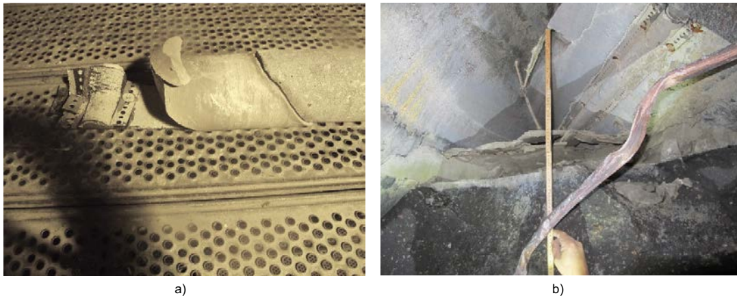
Figure 6-8. a) Drill core “centre” and b) void on top of the concrete.
