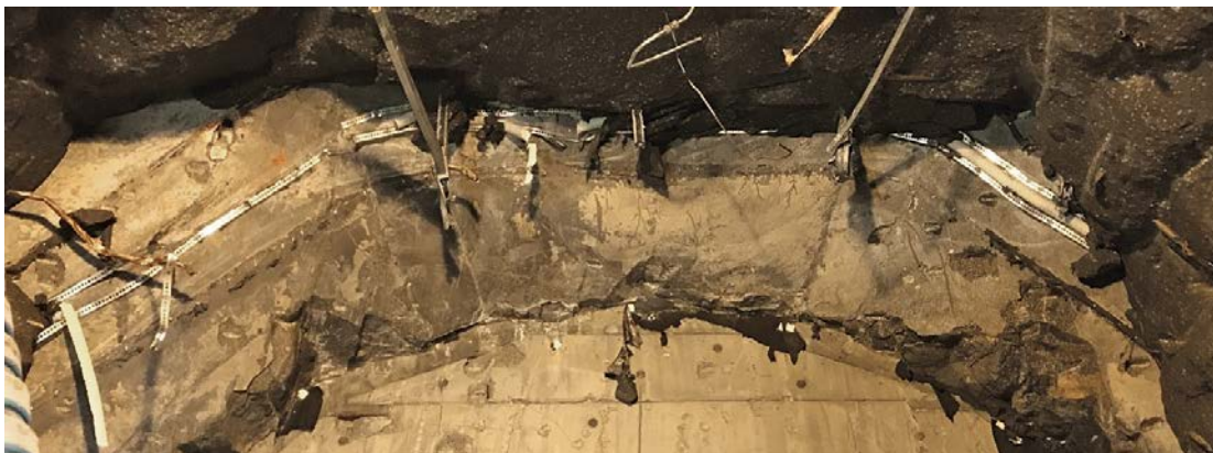
Figure 7-9. Some areas are visible with a thin layer of grout on the upstream side of the slot.
