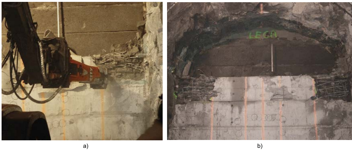
Figure 7-14. a) A hydraulic hammer was used on both ends of each concrete beam to crush the concrete. b) After crushing the concrete at both ends the steel anchoring to the rock was cut and the beam could then be lifted away by a large loading machine. From Åkesson et al. (2019).
