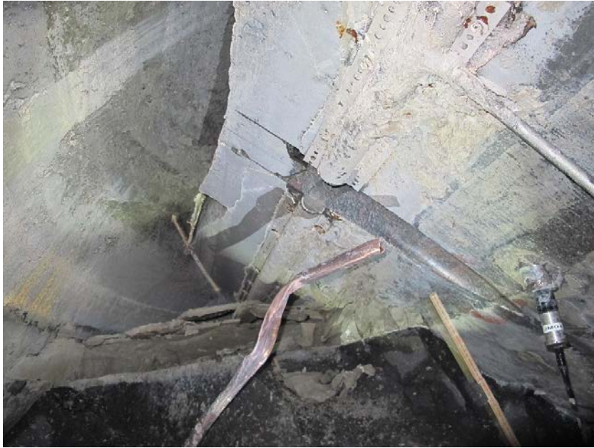
Figure 7-12. Photo of the void and the joint-meter JM01 to the right.
