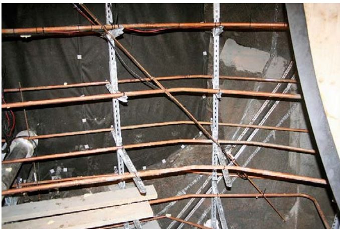
Figure 2-12. Cooling pipes mounted on frame with the grouting tubes visible in the background.
