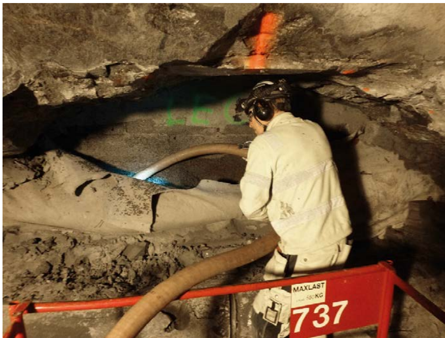
Figure 7-17. A vacuum truck was used to remove the filter material. From Åkesson et al. (2019).
