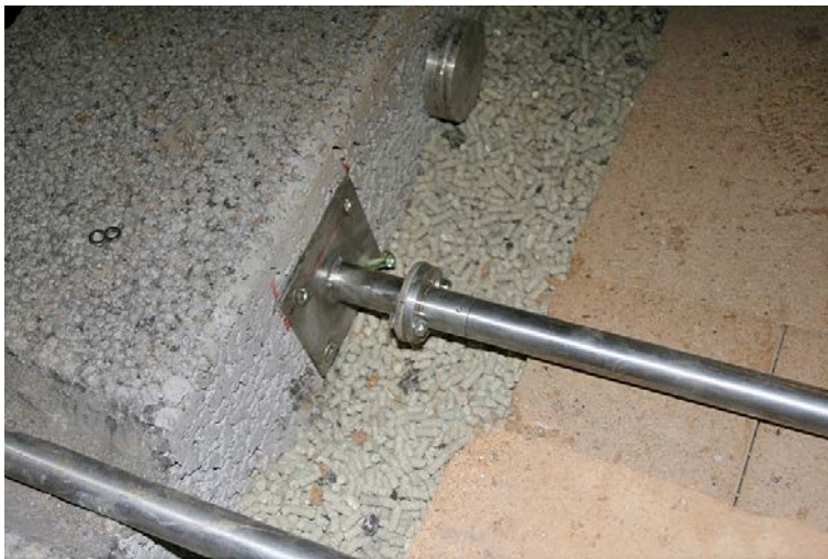
Figure 2-17. An extensometer and a total pressure sensor during the installation of the backfill.
