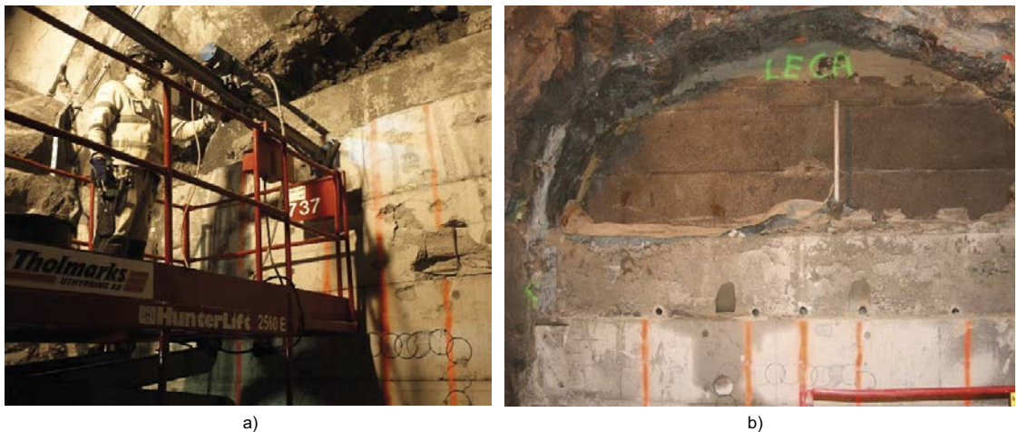
Figure 7-15. a) A scissor platform was used during sampling of the bentonite. b) The exposed bentonite has been sampled. From Åkesson et al. (2019).
