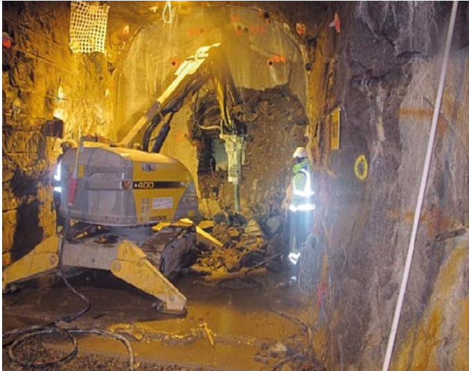
Figure 7-5. Demolition Robot BROKK 400 and the concrete dome after the first day of demolition.
