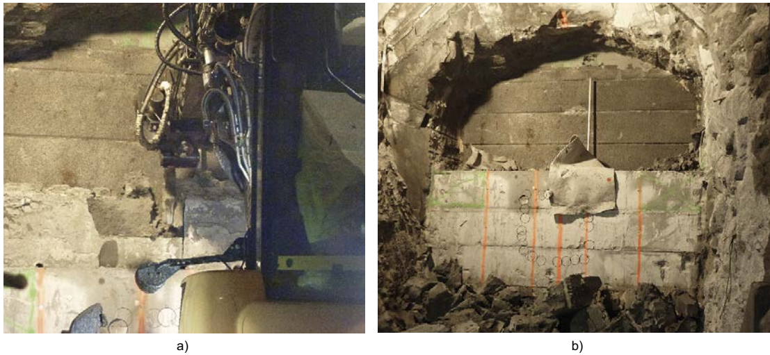
Figure 7-16. a) A special “hook” was used to remove the remaining bentonite above the next concrete beam. b) The main part of the bentonite has been removed, leaving the outer parts close to the rock wall for sampling. From Åkesson et al. (2019).
