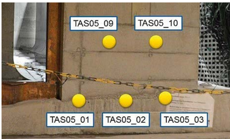
Figure 1-2. Positions of the drilled cores (yellow circles, diameter of 10 cm). TAS05-09 and TAS05-10 drilled cores correspond to Section 2 (truck #2) concrete.
