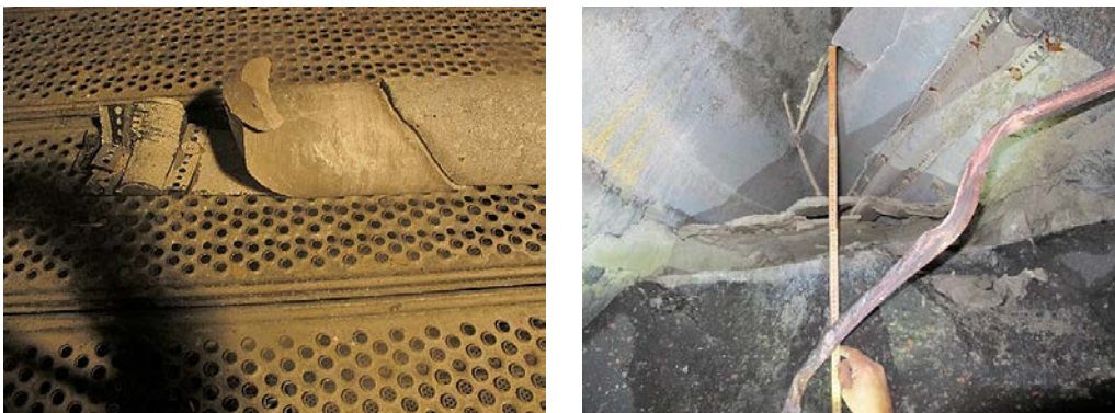
Figure 2-6. Drill core “center” (left) and void on top of the concrete (right).
