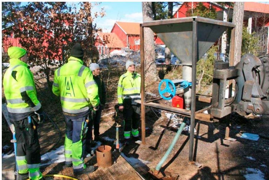
Figure 9-1. The hopper filled with sand is positioned above the borehole. A valve is used to adjust the installation speed. The sand is led from the hopper to the borehole via a flexible tube.
