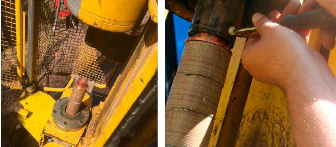
Figure 12-8. A bentonite package is lowered down in the borehole and then connected to the drill tube with the shear bolts.
