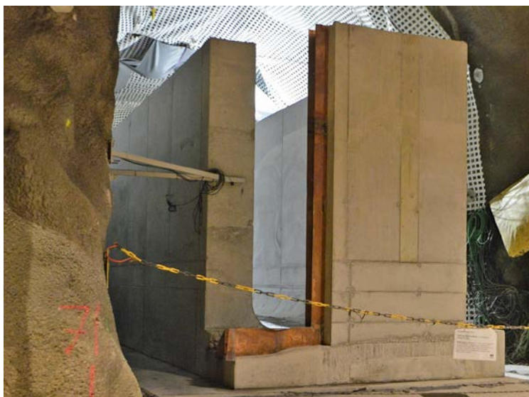
Figure 3-16. An overview image of section 1 (left part) and section 2 (right part) just after demoulding of section 2. The horizontal joint seal in the bottom slab and the vertical joint seal in the wall of section 2 are clearly visible.
