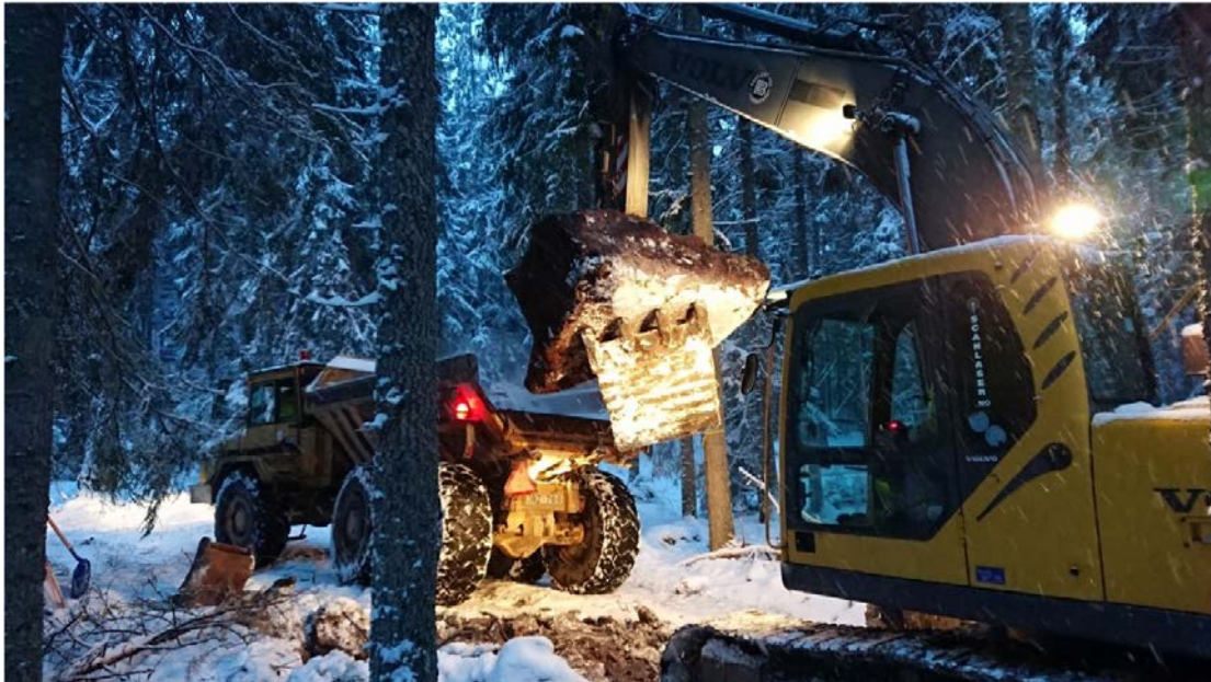
Figure 3-2. Smaller block representative of the RFM045 rock domain being prepared for transport to Sandvik.
