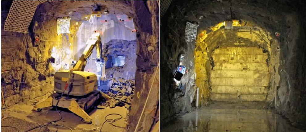
Figure 3-7. Machine for breaching (left) and result after removal of the concrete dome (right).
