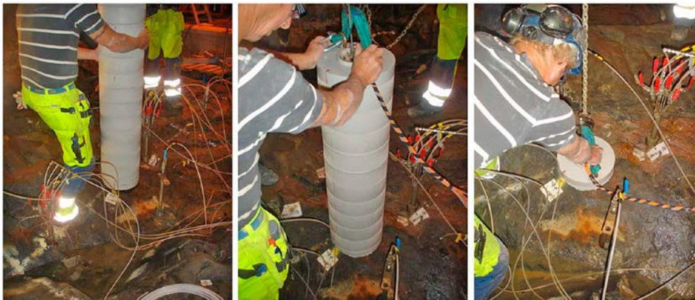
Figure 2-9. Installation of the bentonite blocks in KO0017G01. Photographs are reproduced from Vidstrand et al. (2017).
