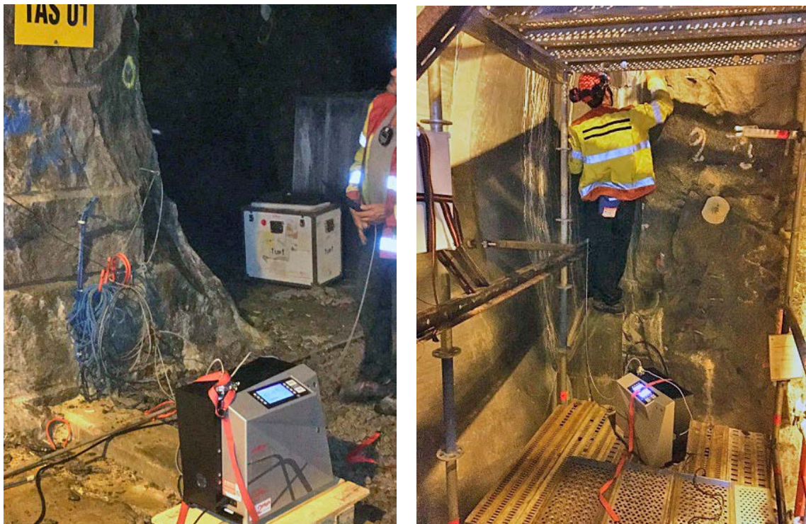
Figure 3-4. Photographs from sniffer leak search; equipment (left) and investigation from scaffold (right).
