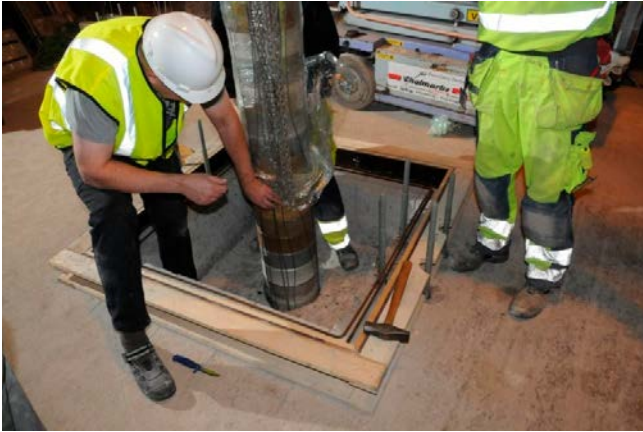
Figure 10-5. The plastic wrapped around the blocks was removed in conjunction with the installation.
