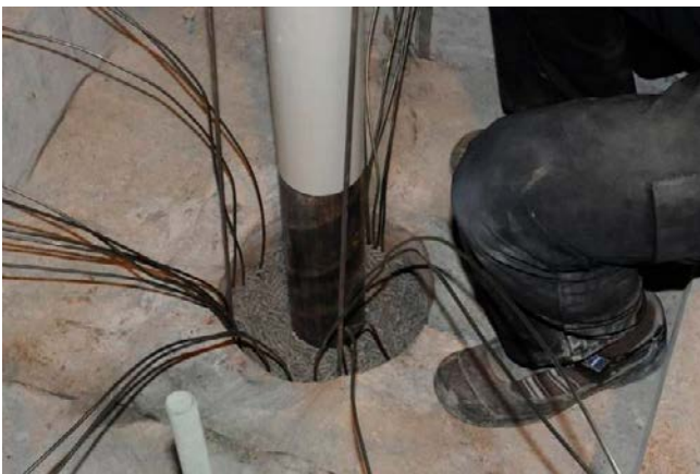
Figure 10-6. The gap between the uppermost block and the rock together with some additional centimetres above the block was filled with bentonite pellets.
