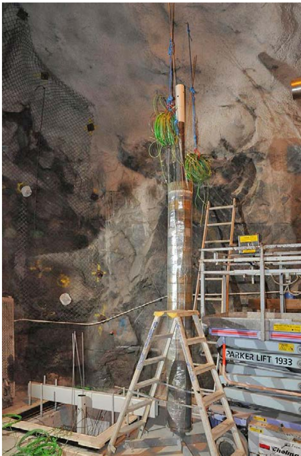
Figure 10-2. The central steel tube is mounted on a platform above the test-hole and the mounting of blocks and sensors have started.
