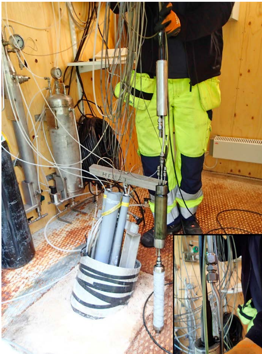
Figure 2-3. The pumping equipment (GEOPUMP UV-45) used for pumping in wide standpipes. It consists of a filter and a pump connected to the mini-packer. The small diameter plastic hose is used for expanding the packer and the plastic hose connected to the pump is the pumping hose (enclosed picture right lower corner).
