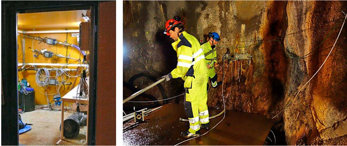
Figure 3-2. Measurement container (left) showing valves, gauges and logger and work at the borehole K03009F01 when changing test section position (right).
