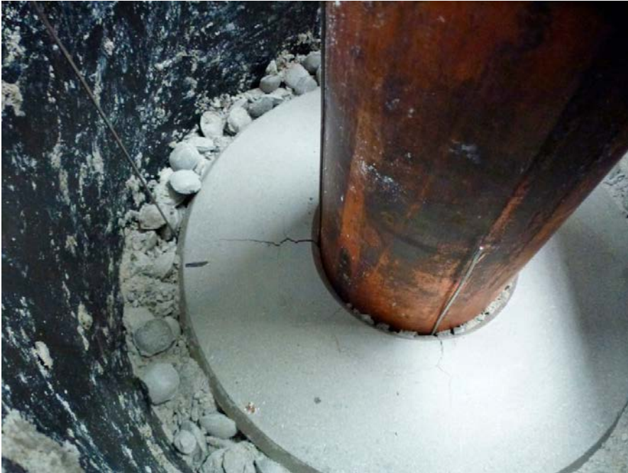
AI-11. Block R1 before the heater was removed. Several cracks are visible although not opened.
