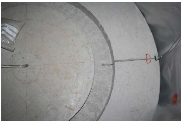
Figure 4-9. The bottom block (C1) in the deposition hole. Note the groove for the bottom of the canister and the installed sensors.
