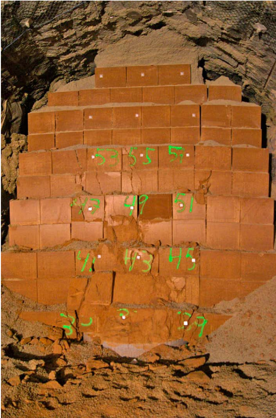
Figure 2-7. Photo of the block stack above the simulated deposition hole taken during excavation showing the displacements of the blocks and cracking of some of them.
