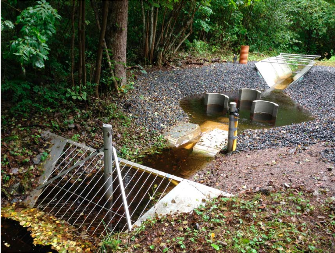
Figure 2-3. The refurbished PFM002669 station, with a pool and parts of concrete pipes between the two flumes, reducing the approach flow velocity towards the large flume. The picture also shows the grating and the attached tube hosting the EC and temperature sensors, some distance upstream of the small flume. During 2016, it is planned to construct a cottage above the large flume.
