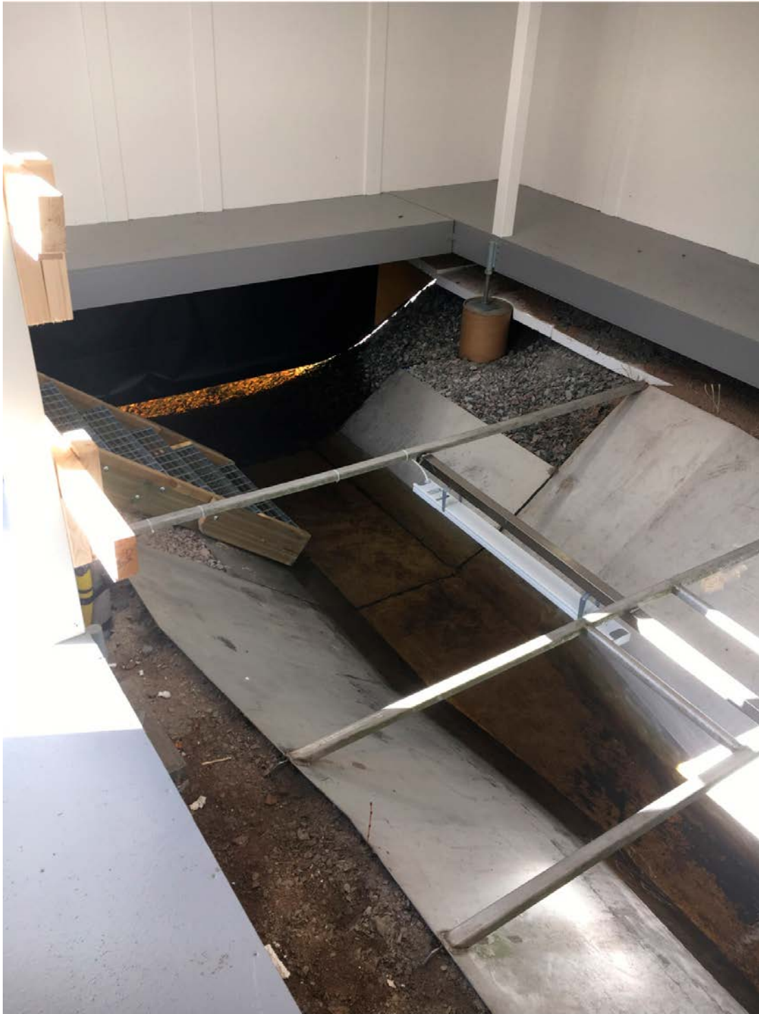
Figure 2-5. Interior view of the cottage, showing one of the infra heaters and the walking platform that improves working conditions at field inspections.
