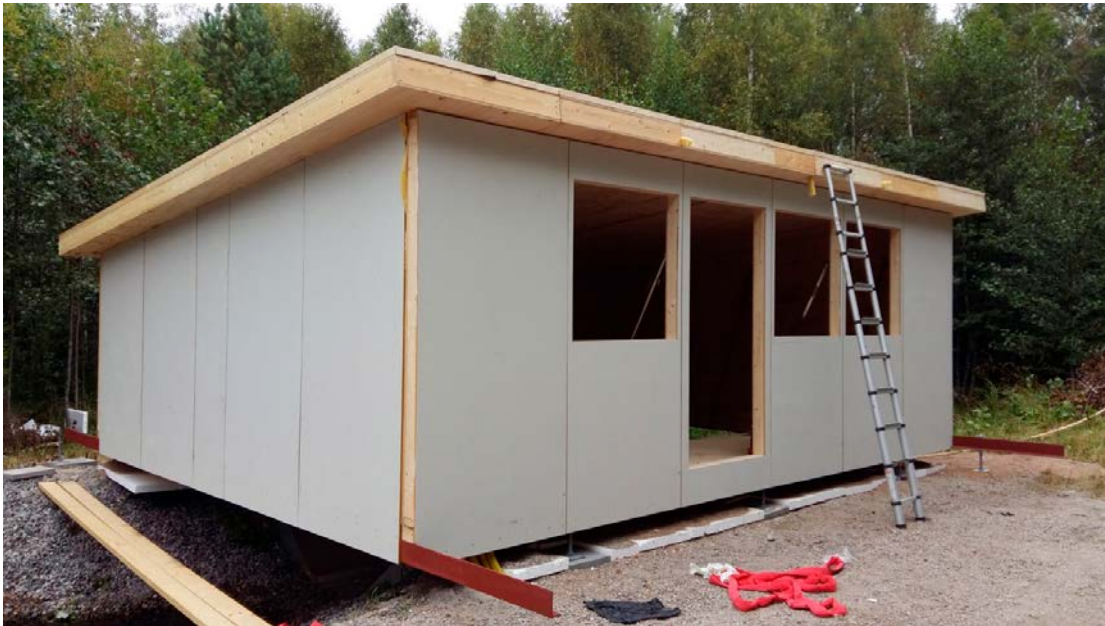
Figure 2-4. Ongoing construction of the cottage above the large flume at PFM005764 during autumn 2015.
