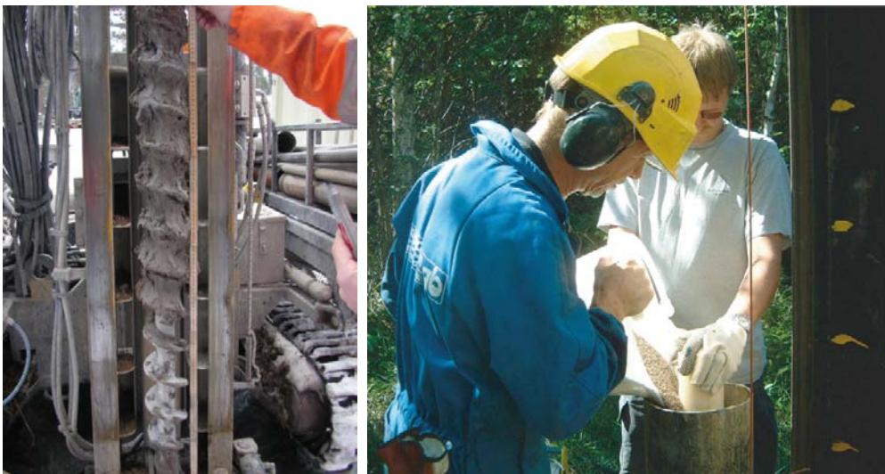
Figure 6-19. Auger drilling was used during installation of the monitoring wells (left). The right picture shows installation of the HDPE well screen, riser pipes, sand filter and bentonite sealing in a groundwater monitoring well inside a temporary steel casing. The snap-shot illustrates the bentonite being emplaced between the riser pipe and the temporary steel casing used to facilitate the filling.
