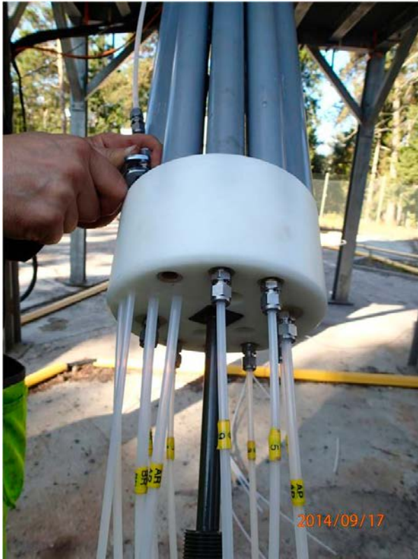
Figure 4-28. PEEK installation in KFM08D. This specific part is lowered into the borehole and installed at a depth of about 40 metres.
