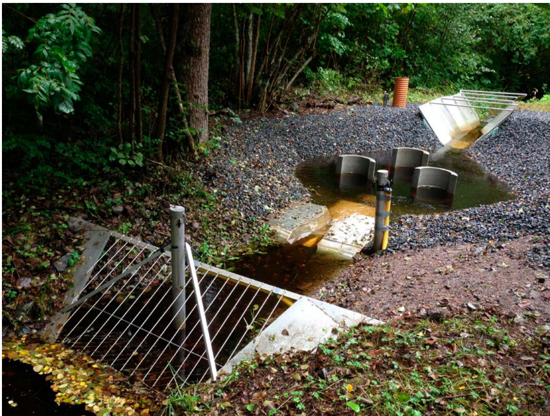
Figure 5-5. The two flumes at the recently (2015) refurbished PFM002669 stream-gauging station.
